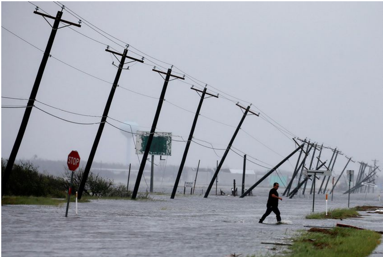
Figure 5-1. Distribution lines in Rockport, Texas following Hurricane Harvey (Reuters 2017)
