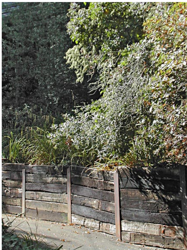
Figure 7. Salvaged creosote-treated railroad ties, now being used in a residential retaining wall.
