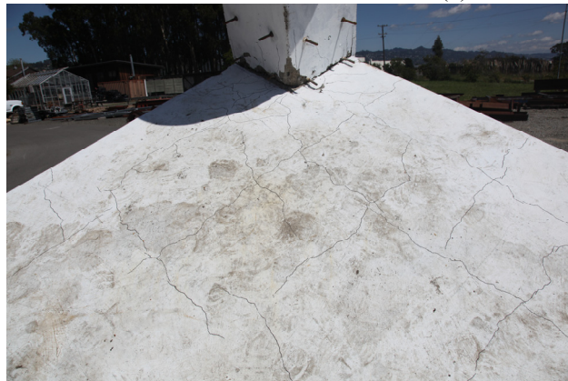
(c) Cracks on slab
