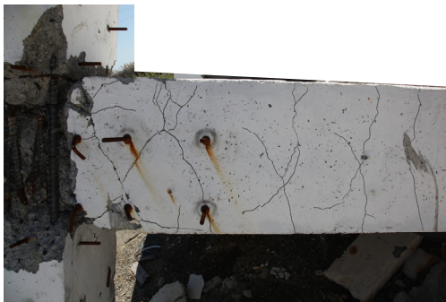
(a) Cracks in EW beam
