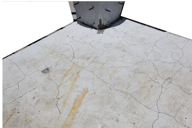
(c) Cracks on slab
