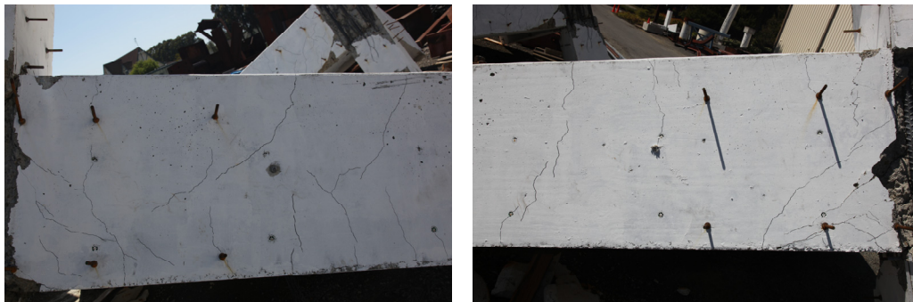
(a) Cracks in EW beam
