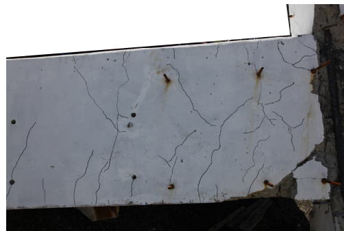
(b) Cracks in NS beam
