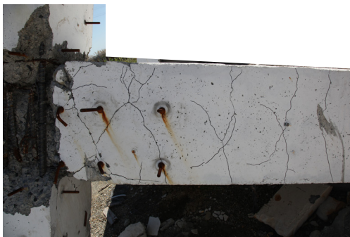
(a) Cracks in EW beam
