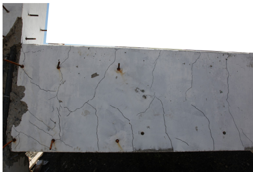
(a) Cracks in EW beam
