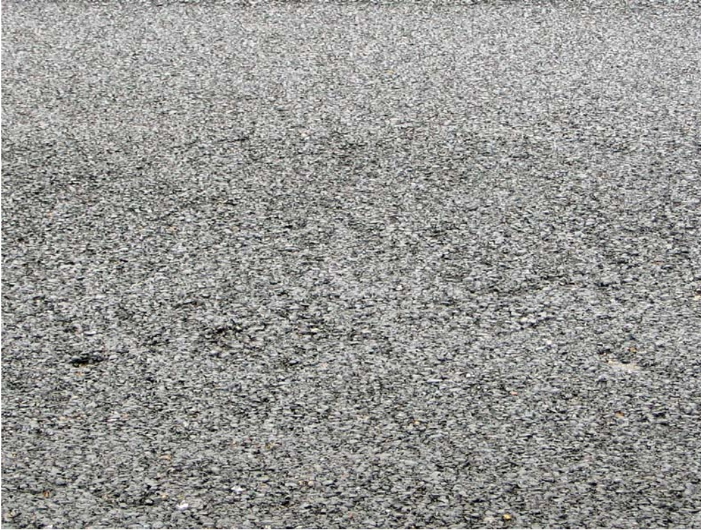
Figure 24. Raveling at Station 56+80 (northbound direction).
