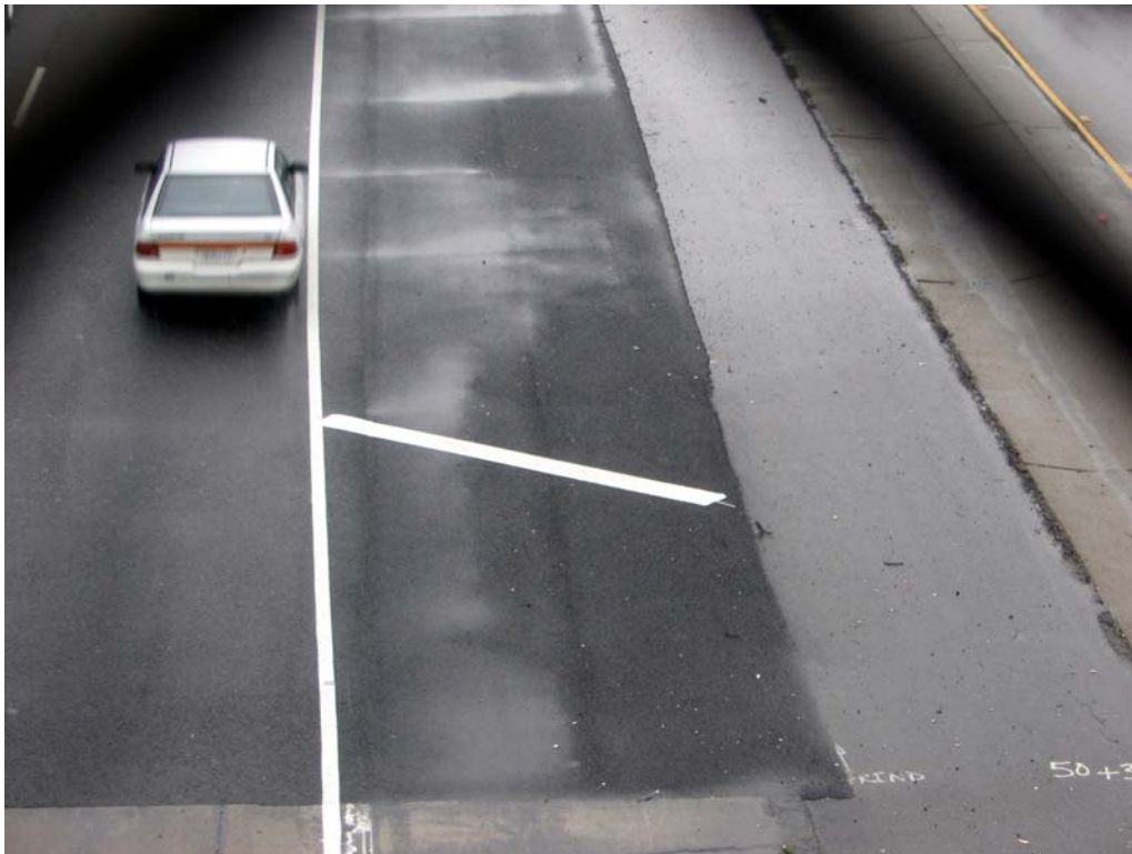
Figure 17. Ponding at Station 50+00 (outside lanes, northbound).
