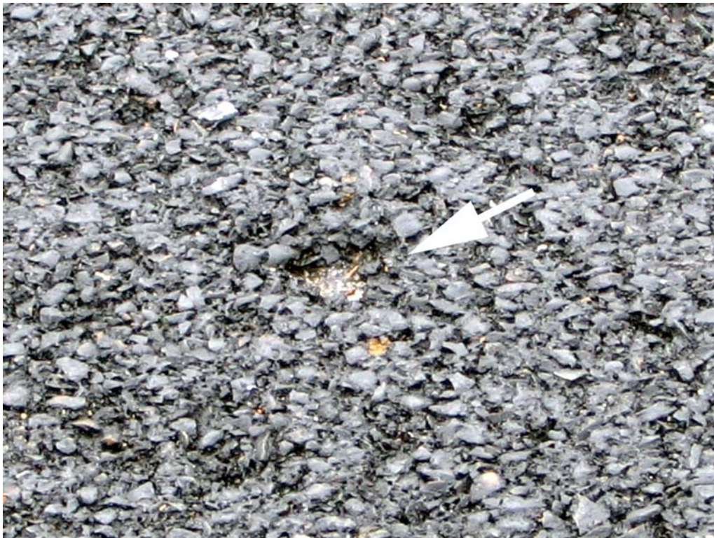
Figure 23. Hole at Station 56+80 (northbound direction).
