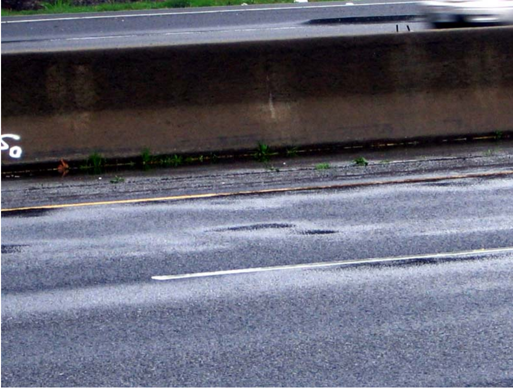
Figure 11. Ponding at Station 51+60 (inside lanes, southbound).
