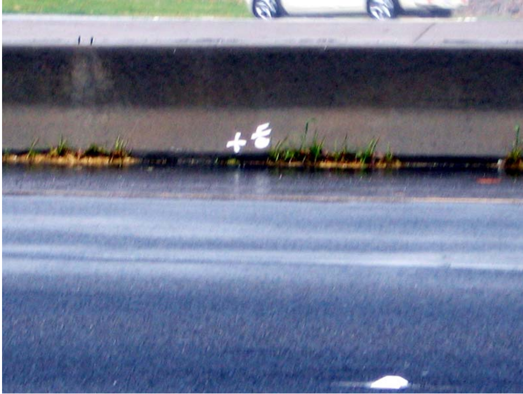
Figure 7 . Ponding at Station 50+40 (inside lanes, southbound).
