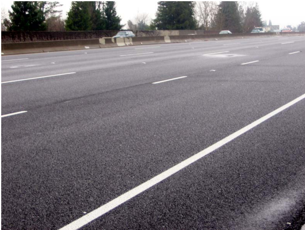
Figure 21. Ponding between between Station 54+00 and 56+00 (inside lanes, northbound).
