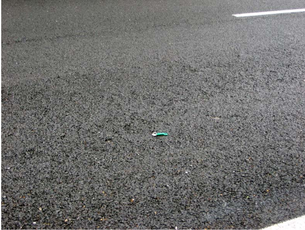
Figure 22. Raveling at Station 56+80 (northbound direction).
