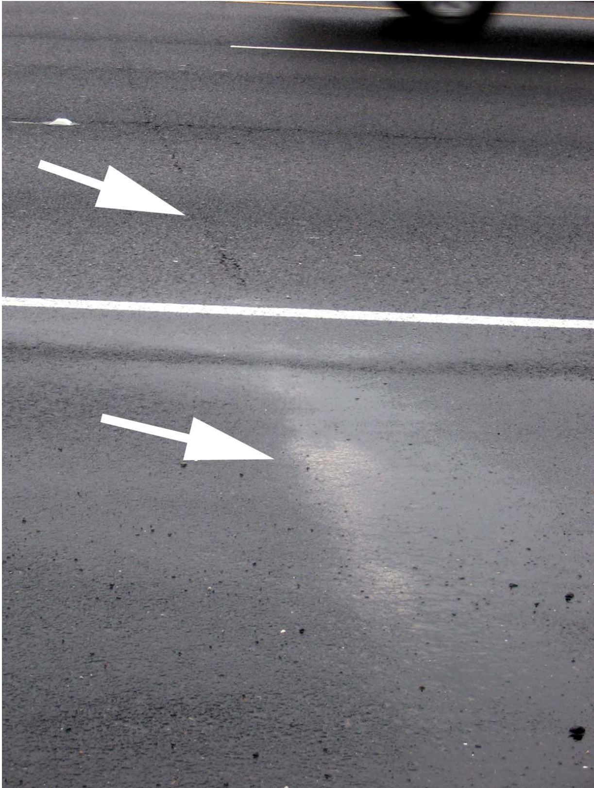
Figure 15. Reflection cracking and pumping of fines between Station 52+00 and 53+00 (northbound lanes).
