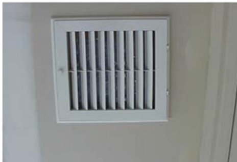
Filter Backed Grill Covering the OA Intake
