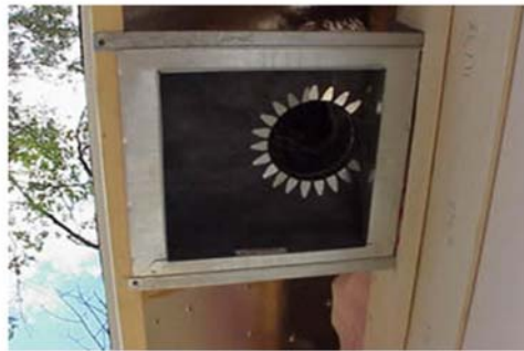
OA Intake Duct in Soffit
