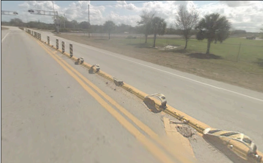
1 2 FIGURE 4 Damage to Channelization Devices in Frostproof, Florida 3
