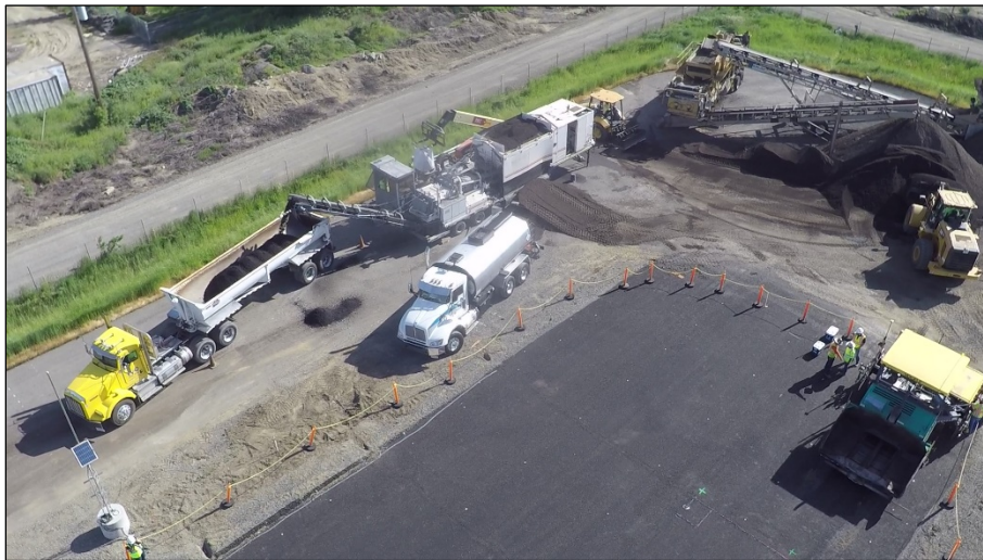
Figure 3.22: CCPR: Central plant setup.
