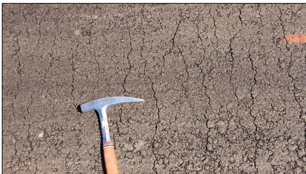
Figure 3.27: CCPR: Shear cracks after pneumatic tired roller passes.
