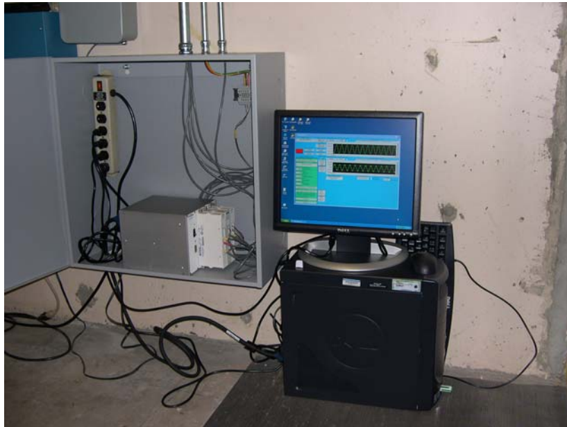
Figure 9 PPSM Monitoring Unit at BPA's Portland Headquarters
