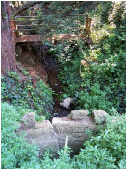
photo: facing downstream, cracked wall and bridge
