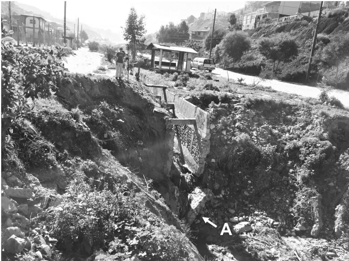
Figure 8. SW concrete flume facing upstream where portions of the concrete sides and bottom collapsed due to excess incision and widening. Fallen concrete pieces labelled (A).
