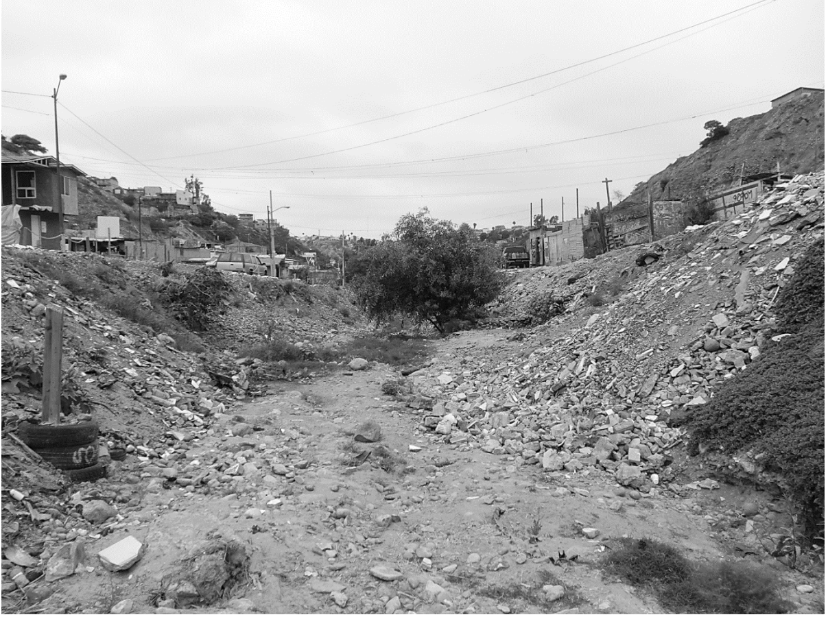
Figure 4. Residents fill in the channel with loose sediment and construction debris to prevent the channel from eroding into their homes. Picture taken in the SW channel.
