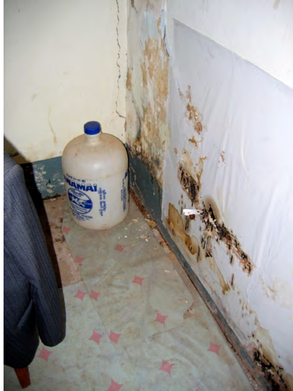
Figure 3.8: Mineral deposits and mold on the rear interior wall of Vannasin’s Technical Department, indicating where floodwaters seep through the walls and into the room during the rainy season.
