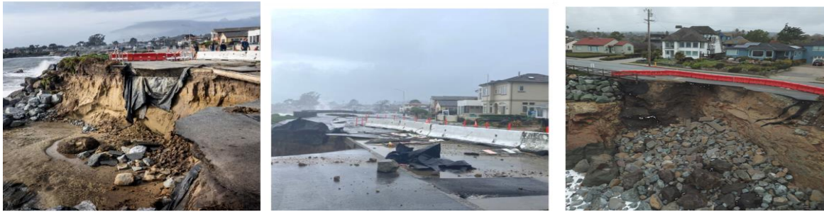
FIGURE 6 IMAGES OF THE JANUARY 2023 COASTAL STORM IMPACTS ALONG WEST CLIFF DRIVE, SANTA CRUZ, CA.
