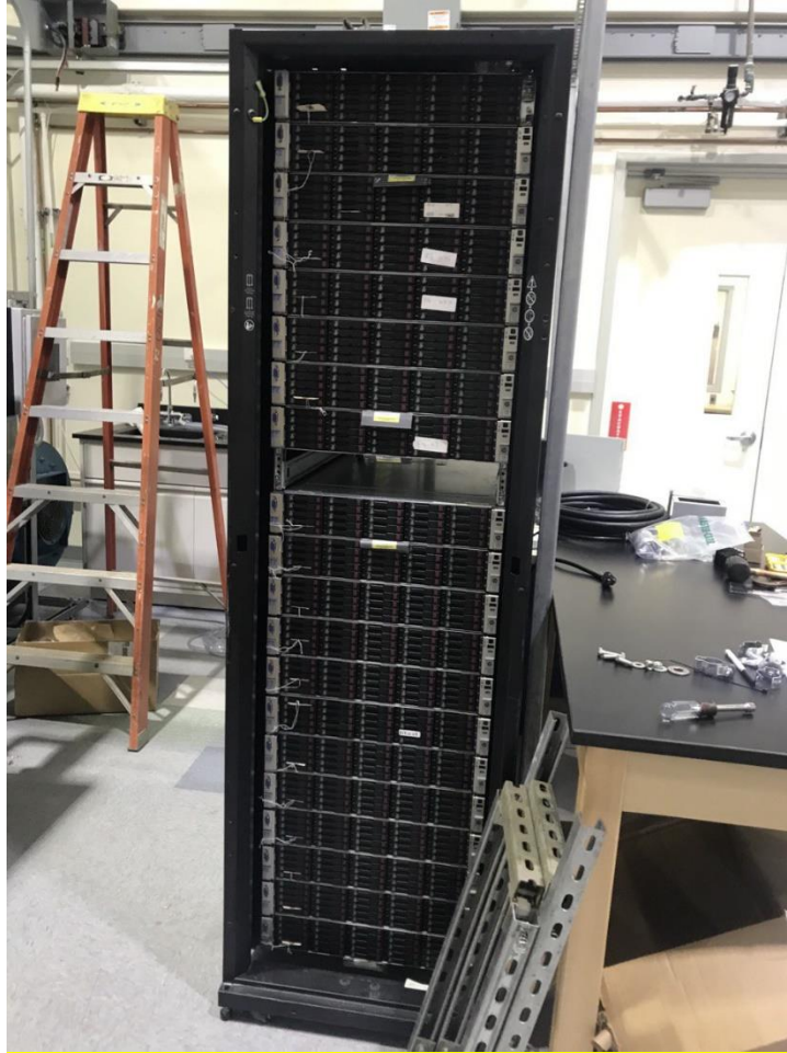
Figure 92. Server rack at NFCRC laboratory
