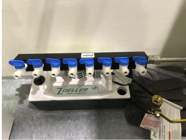
Figure 90. Manifold and valves for fuel cell supply water.
