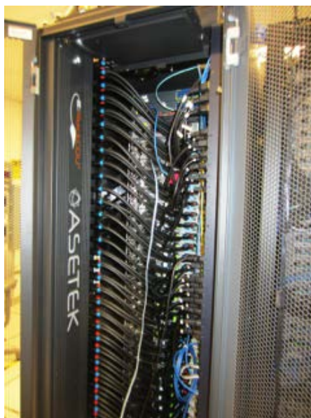
Figure 2.8.1: Asetek system supplying liquid to IT equipment
