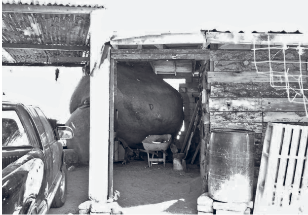
Figure 8. Granitic boulder supporting the roof of Gloria Regino Arballo's garage (photo courtesy of Everardo Garduño).
