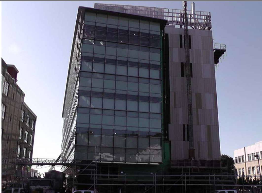
Picture 3 East facade of the Helios building with the beginning glazing façade.
