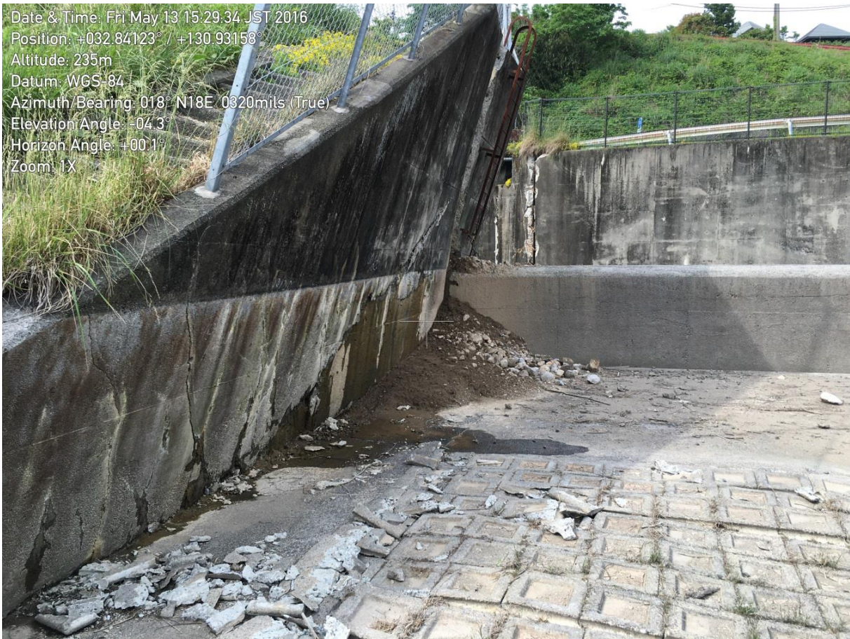
Fig. 2.6. Soil intrusion into the spillway due to fault movement that opened up a gap in a retaining wall of the Oh-Kirihata Dam. Image courtesy of NSF-Sponsored GEER Report #GEER-048 (Kayen et al. 2016).
