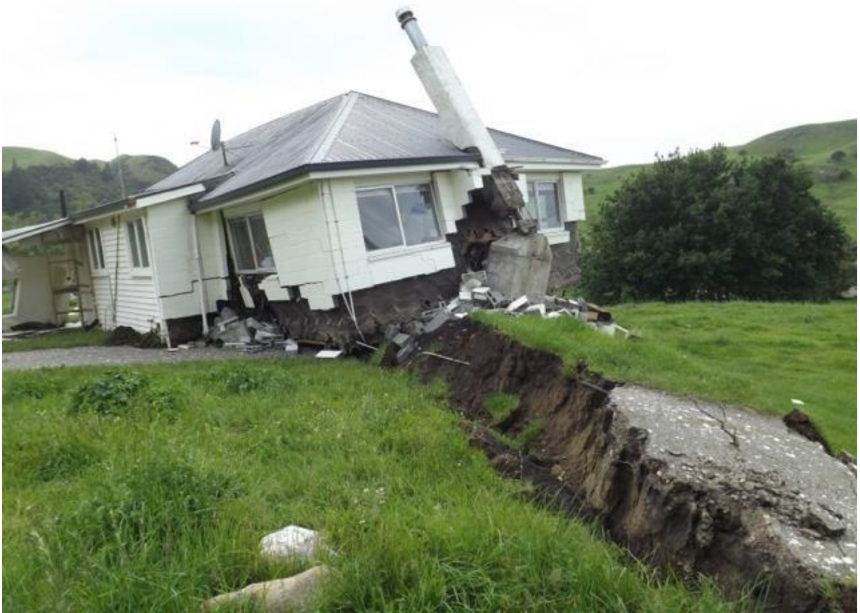
Fig. 2.13. Single-story home next to the Kaikoura coast damaged by reverse fault surface rupture from the 2016 Kaikoura, New Zealand, earthquake (from Stirling et al. 2017, reproduced with permission of the New Zealand Society for Earthquake Engineering Inc.; photo by Tim Little).
