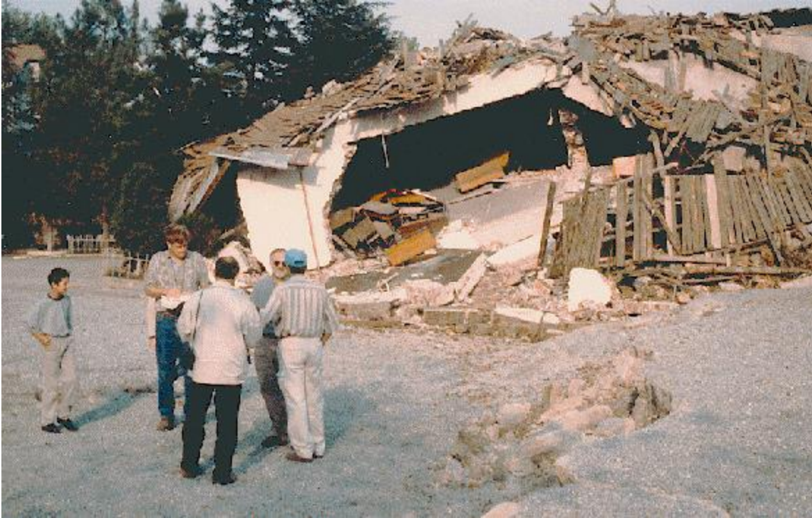
Fig. 1.2. Damage to a primary school building in the village of Kullar due to rupture on the Sapanca fault segment during the 1999 Kocaeli, Turkey, earthquake (Photo by L.S. Cluff; from Lettis et al. 2000, reproduced with permission of the Earthquake Engineering Research Institute). Lettis et al. (2000) report approximately 2 m of lateral offset and 0.5 m of vertical offset at this location.
