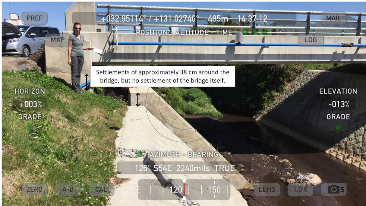
Fig. 2.9. Bridge located across the Aso Caldera Depression Zone that underwent negligible settlement in comparison to the surrounding soil. Image courtesy of NSF-Sponsored GEER Report #GEER-048 (Kayen et al. 2016).
