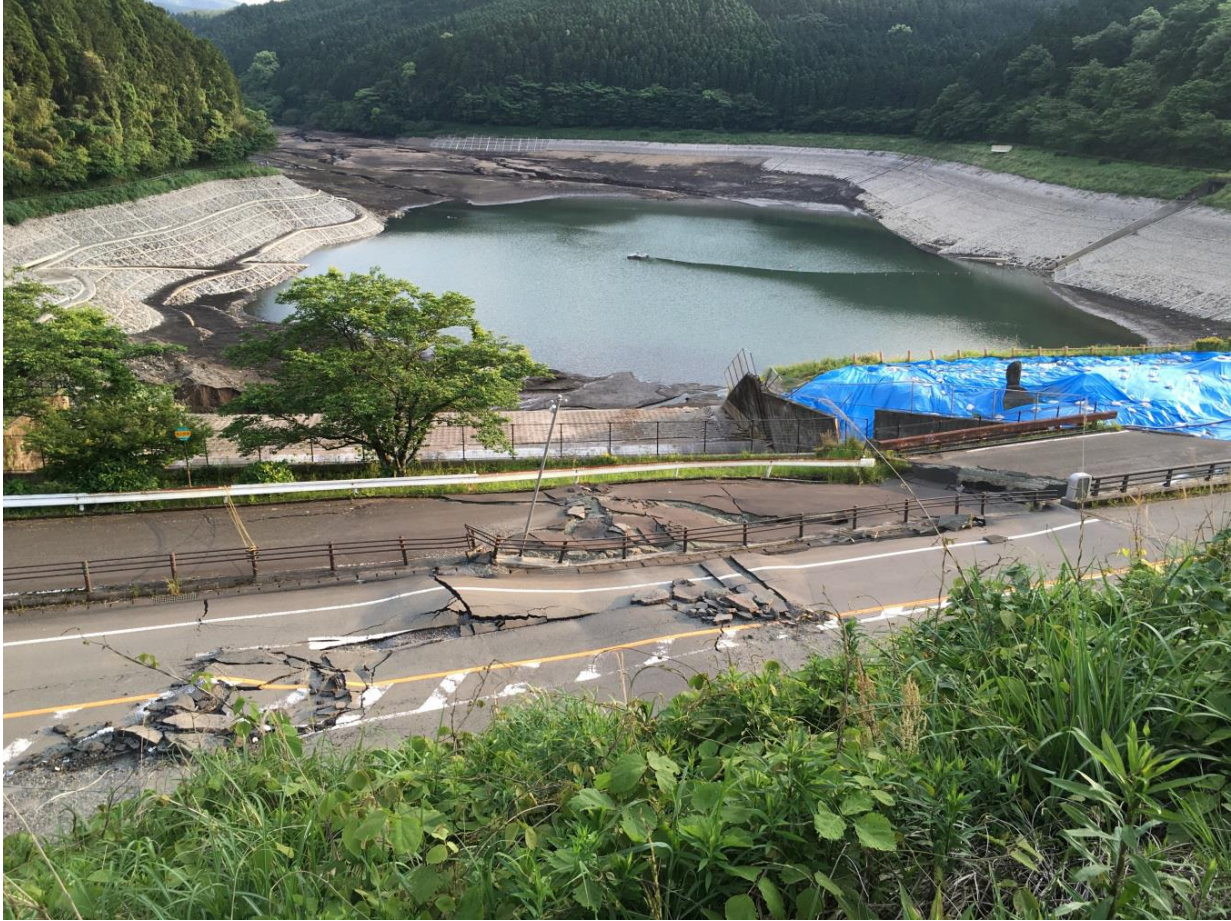
Fig. 2.4. View of a strand of the Futagawa Fault crossing through the Oh-Kirihata Dam after the 2016 Kumamoto, Japan, earthquake. Image courtesy of NSF-Sponsored GEER Report #GEER-048 (Kayen et al. 2016).
