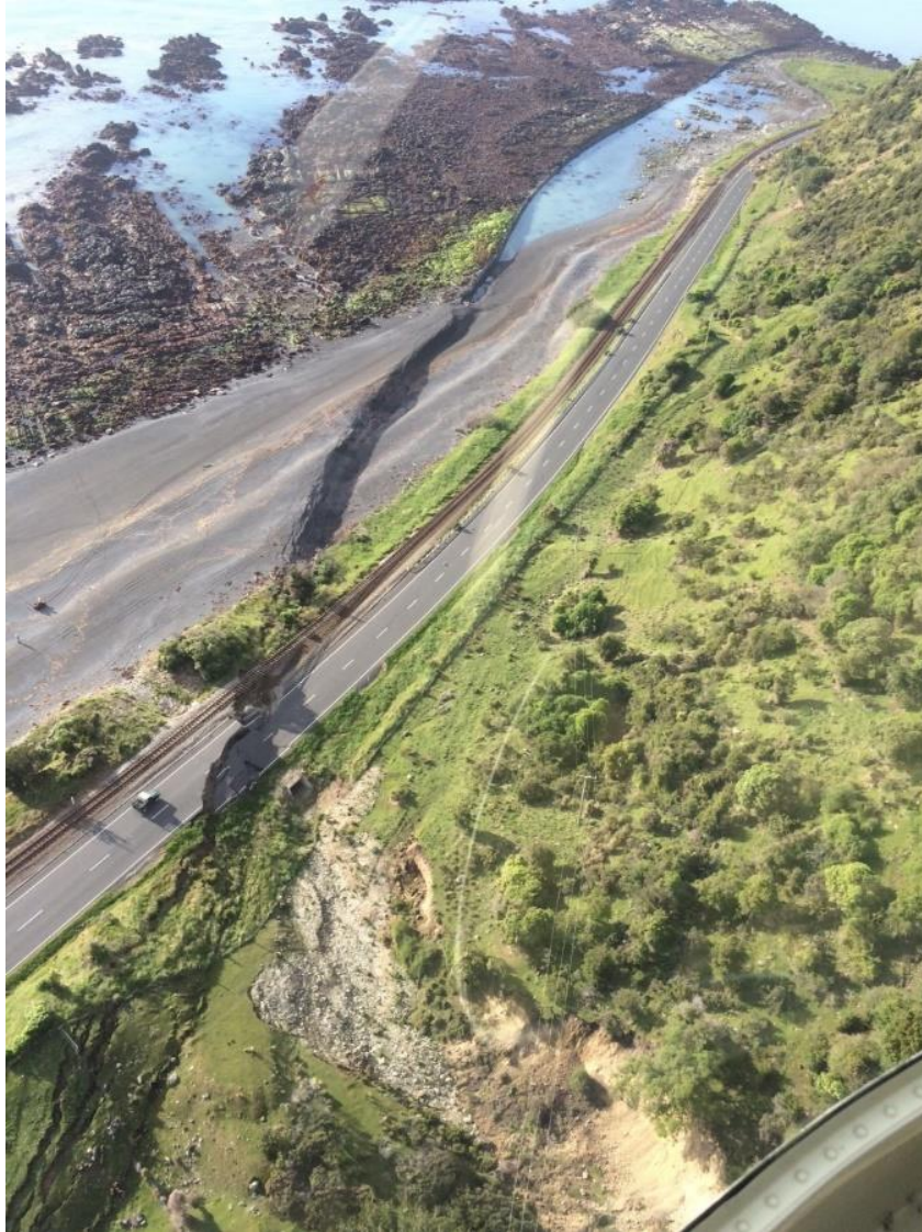
Fig. 2.12. Fault rupture through State Highway 1 in Kaikoura, New Zealand after the 2016 Kaikoura, New Zealand, earthquake (from Stirling et al. 2017, reproduced with permission of the New Zealand Society for Earthquake Engineering Inc.). The exposed seabed is seen at the top of the figure.
