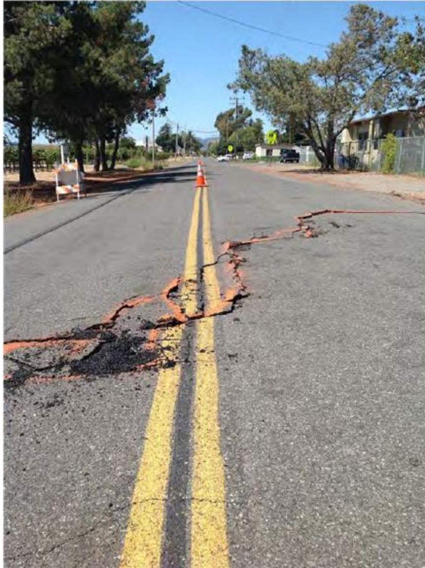
Fig. 2.2. Example of a surface fault rupture trace in asphalt resulting from the 2014 South Napa, California, earthquake. The center lane divider indicates right-lateral offset. Image courtesy of NSF-Sponsored GEER Report #GEER-037 (Bray et al. 2014).
