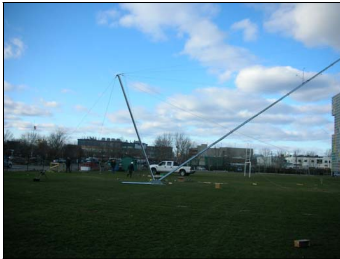
Figure 1: Installation photos from MIT Project Full Breeze Sites 1 and 2
