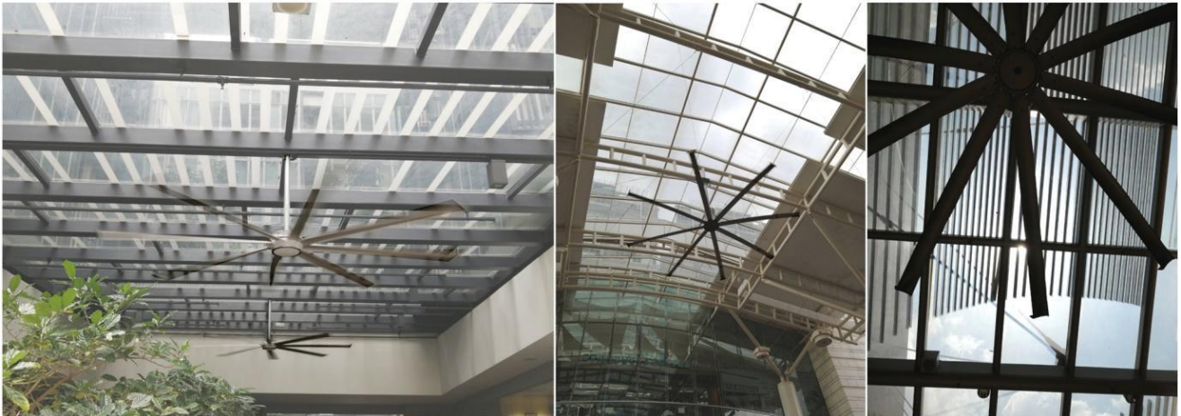
Figure 42. Ceiling fans installed onto skylight applications in Singapore, creating problems of strobing and flicker when daylight is admitted into the space.
