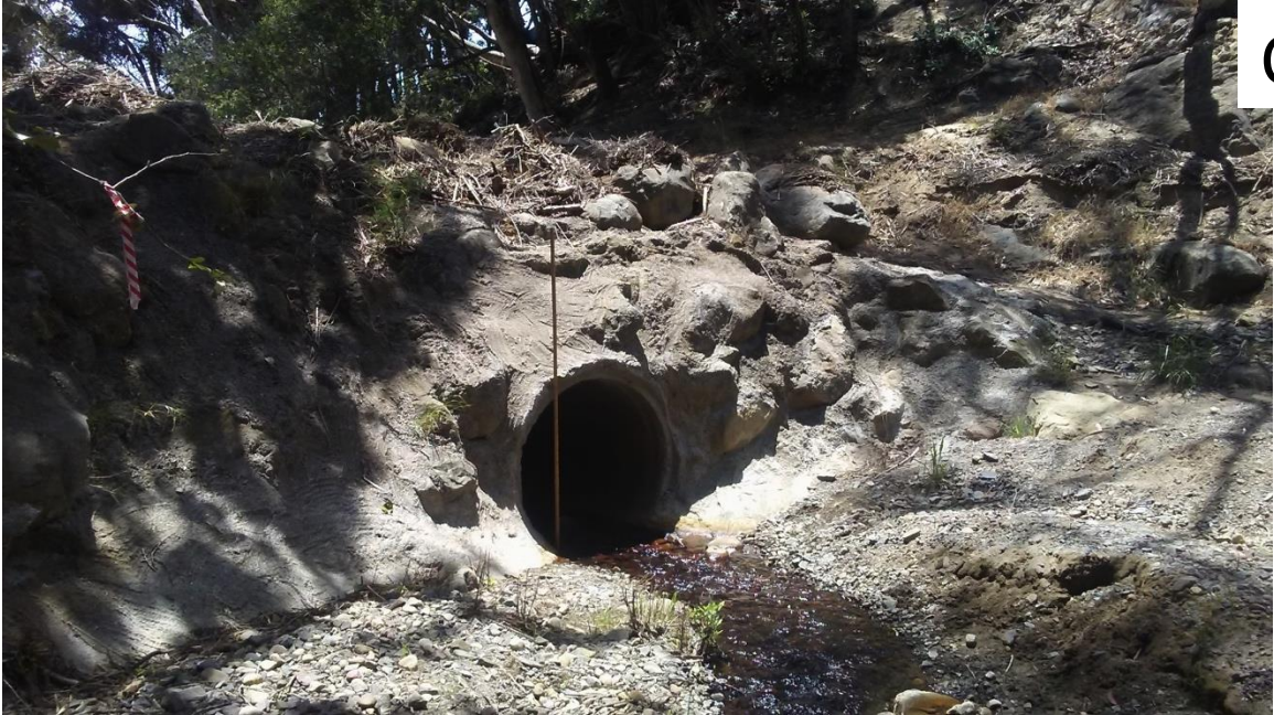
Figure 4: San Ysidro Creek study location (N34°27'24.3"–W119°37'23.4") before (A) and after (B) December 2016 and January 2017 storms. (C) San Ysidro Creek second study location (34°26'58.5"N 119°37'22.3"W).
