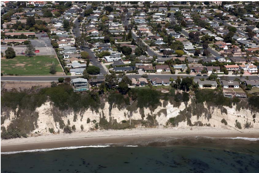
Figure 2.9: A Number of Homes along the Mesa Are within 50 Feet of the Cliff Edge
