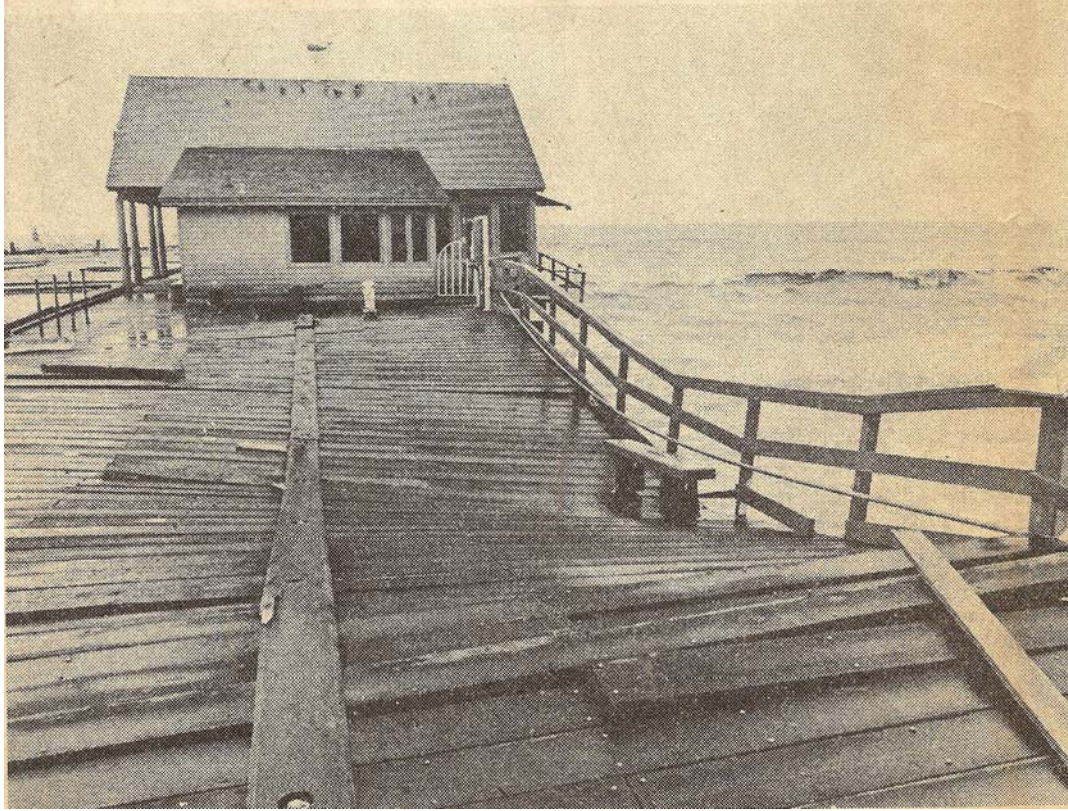
Figure 2.16: The End of Stearns Wharf Sags from a Loss of Pilings in early March 1983 Due to Impacts of Large Waves at Times of High Tides and Elevated Sea Level
