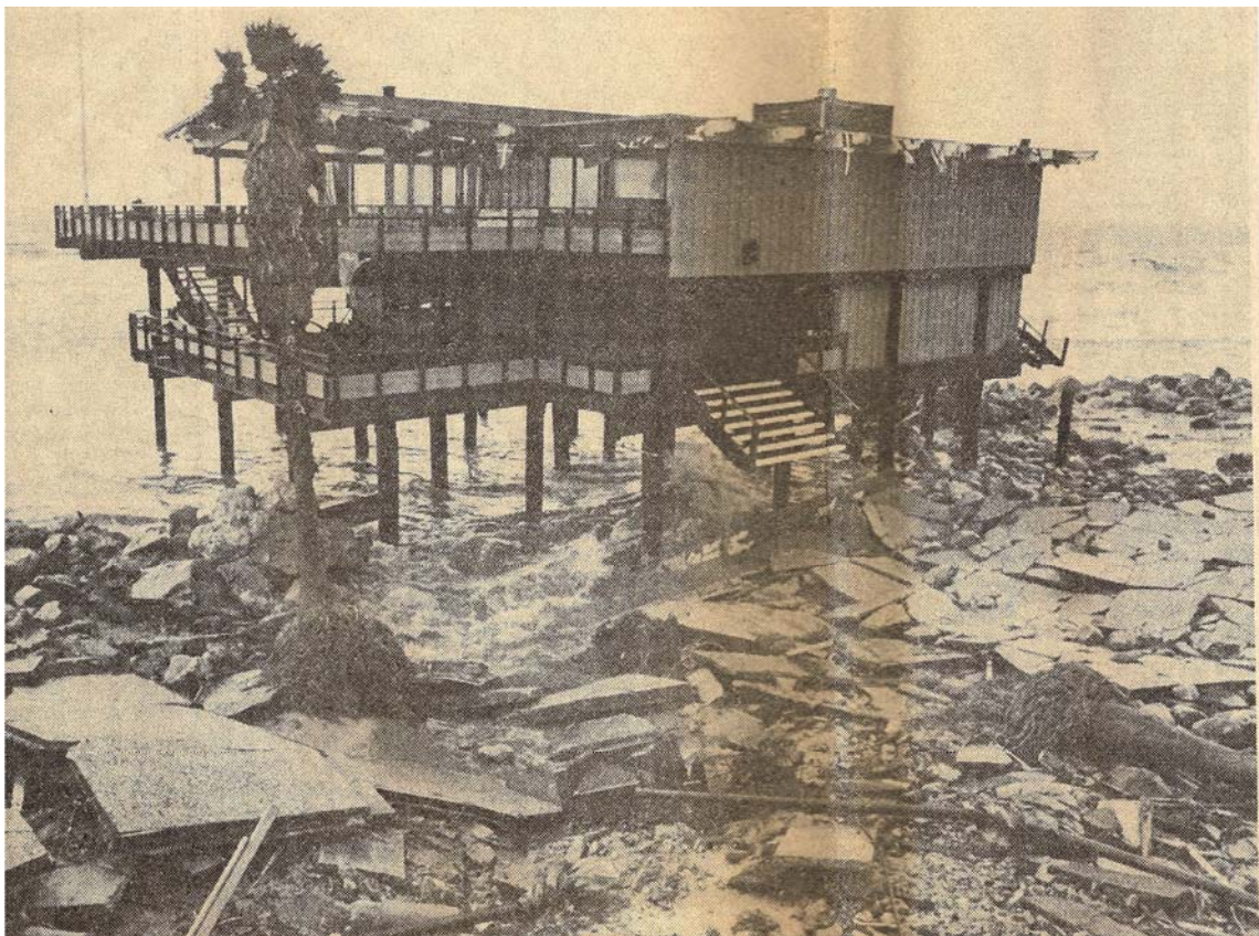
Figure 2.14: Beach Erosion Extended beneath the Santa Barbara Yacht Club in March 1983
