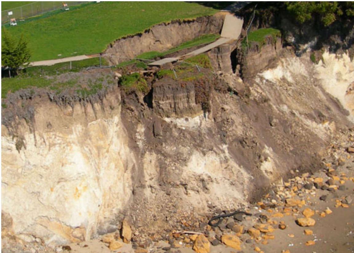
Figure 2.7: January 2008 Landslide along the Cliff at Shoreline Park Moved the Cliff Edge Landward by as Much as 38 Feet and Eliminated a Portion of the Sidewalk
