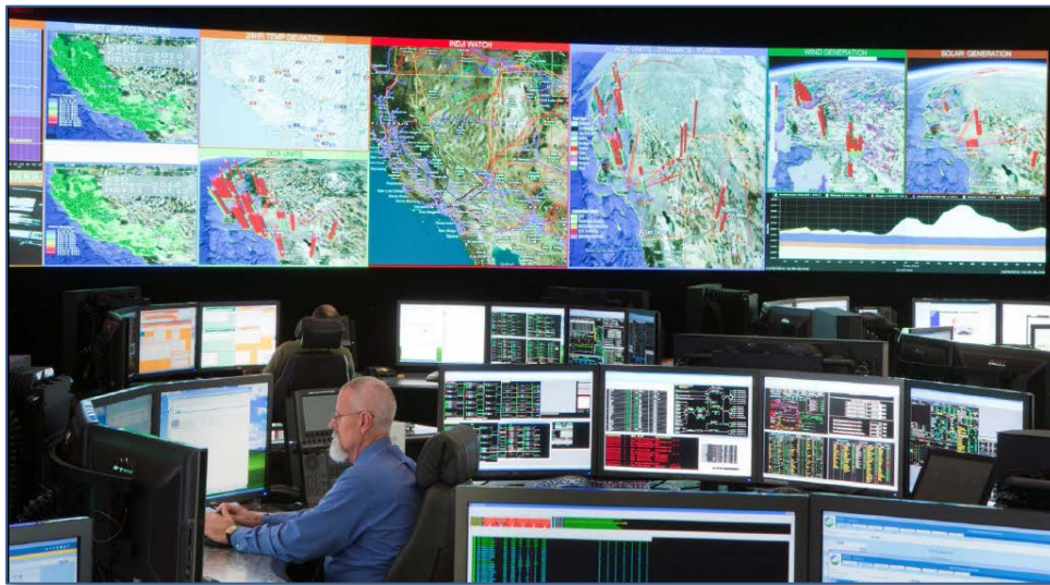
Figure 8: CAISO Control Room Tracking Renewable Profiles
