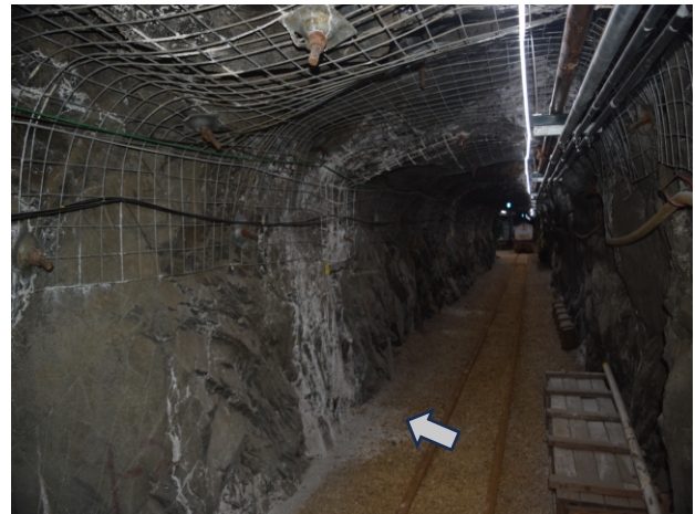
Figure 3b. Weeps in drift are marked by precipitate from dissolved solids in the water entering the drift (arrow points to intersection of a precipitate zone with the drift). The intersection of this fracture on the drift wall (Fig. 3a) can be followed across the ceiling although it does not have a clear expression on the right hand wall in the photograph.
