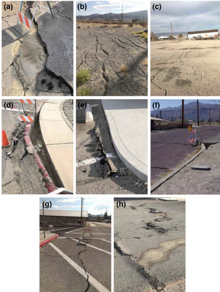
897 898 Figure 6. Ground failure from liquefaction in Trona. (a) Sand boil along a pavement crack 899 created from lateral spreading (35.757483°, -117.37806°). (b, c) Extensional cracks 900 caused by lateral spreading (35.757325°, -117.377705°; 35.75966°, -117.375892°). (d, f) 901 Damaged asphalt from buckled curb edge (35.75936°, -117.37676°; 35.762387°, - 902 117.372586°). (e, h) Compressional features from lateral spreading (35.75897°, - 903 117.37561°; 35.75909°, -117.37552°). (g) compressional and adjacent extensional
