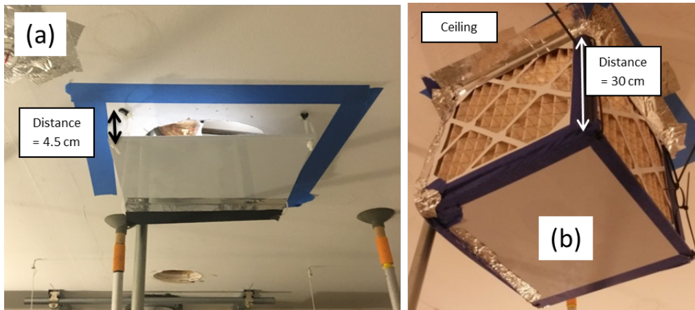
Figure 7. Detail of air inlet: (a) old version; (b) new version (with a ceiling diffuser and MERV 11 air filters)
