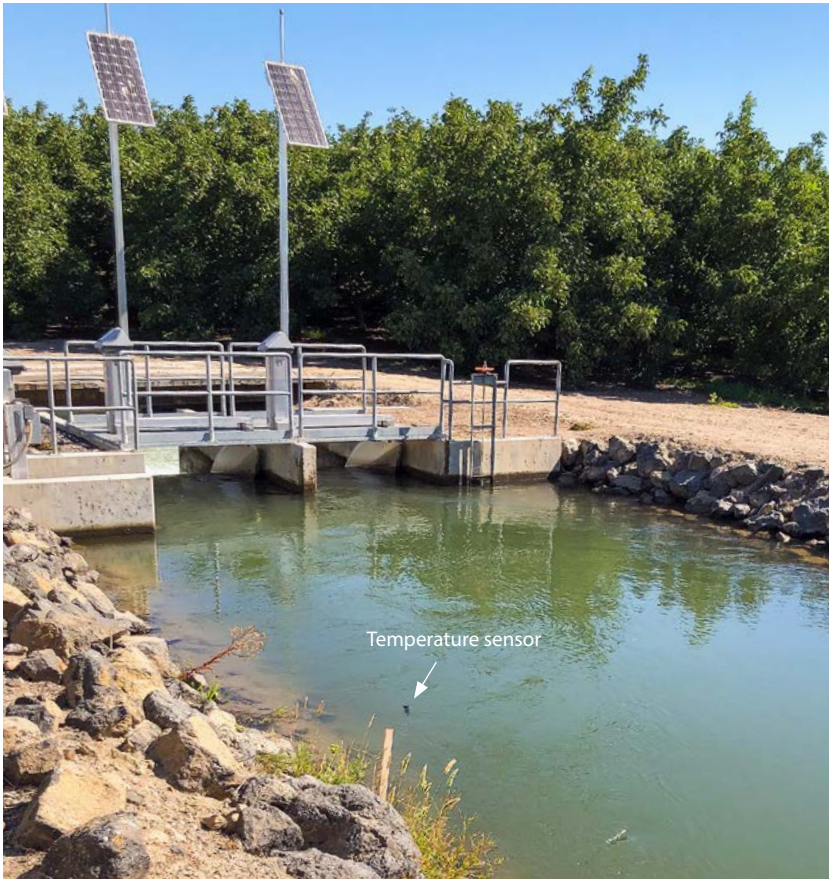
A water temperature sensor visible in the water, near an automated gate (background). Photo: AJ Borba.
