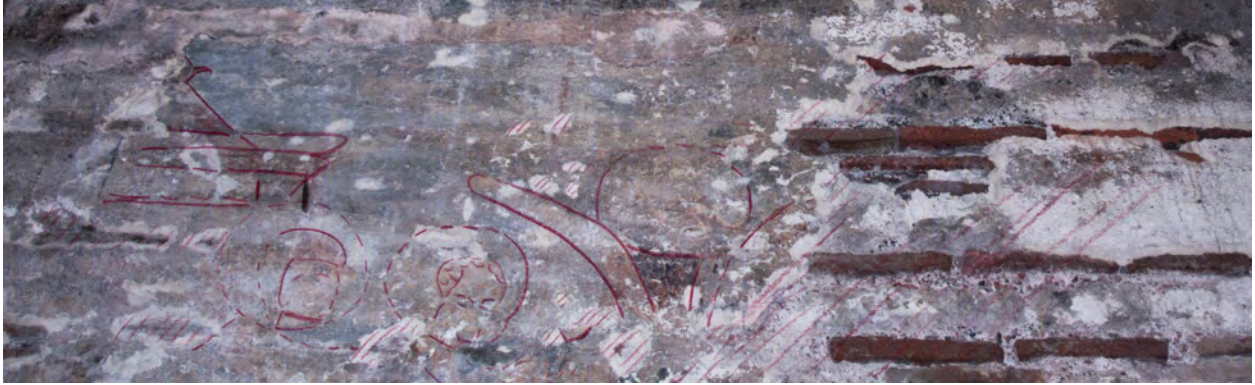
Figure 99: Double-arcade with drawing, West Wall, North Pastophorium, Hagia Sophia, Nicæa (Naomi Pitamber, 2013)
