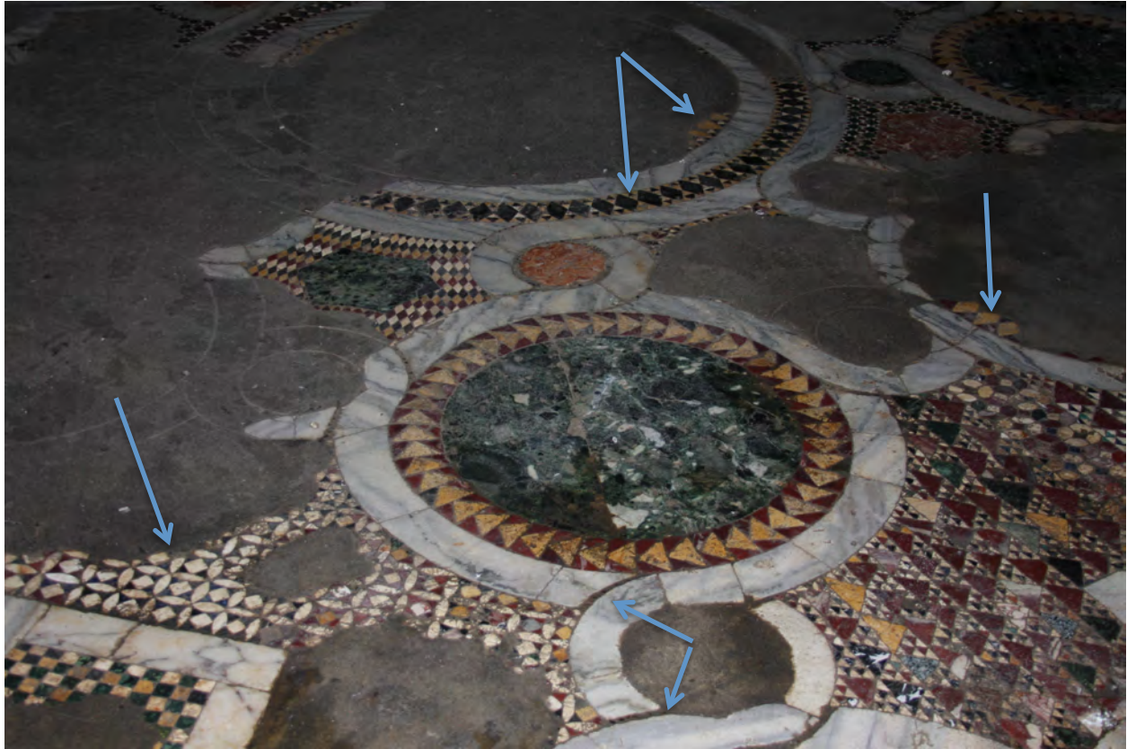
Figure 52: Center disc (missing at top), with double ring of diamond patterned opus sectile , opus tessellatum shading (bottom) and opus sectile pattern, Hagia Sophia, Trebizond (Naomi Pitamber, 2013)
