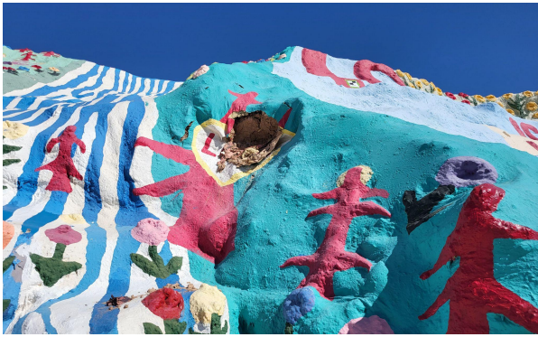
Minor damage on the facade on the southern side of the mountain, caused by hurricane Hilary, Aug. 21, 2023
