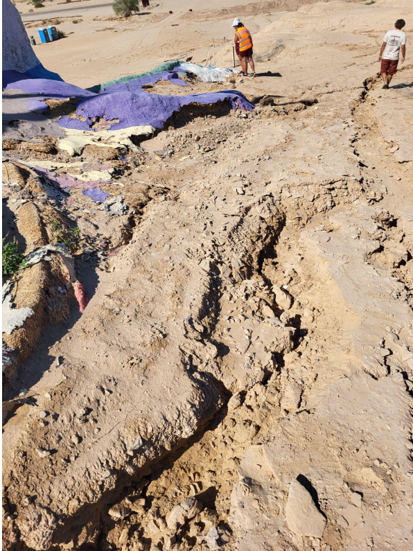
Wash out of the pathway built on the western side, behind the mountain. Caused by hurricane Hilary, Aug. 21, 2023
