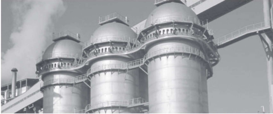
Figure 2-8: Hot blast stove[34]
