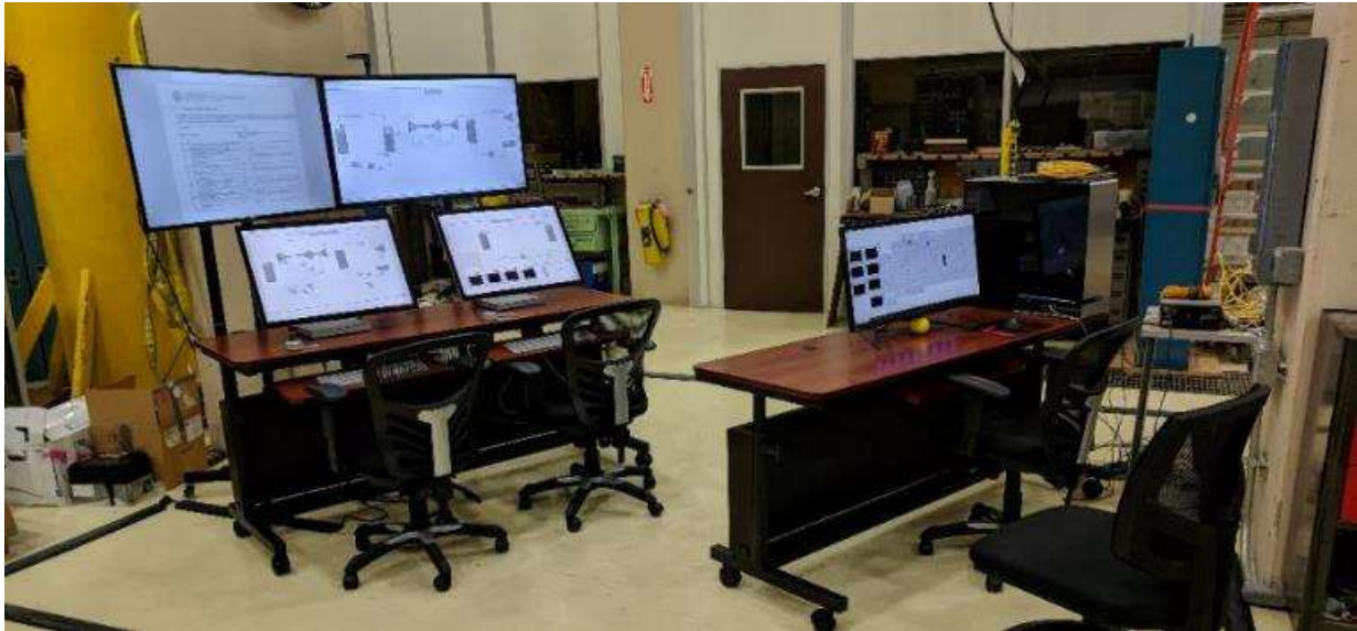
Figure 5-2: ARCO facility consisting of two overview displays, two operator stations (Balance of Plant under the overview panels and on the right and Reactor Operator on the left) and a supervisor station (on the desk behind the operator stations).
