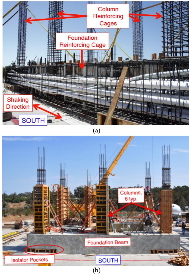
Figure 2.1: Foundation during construction: (a) steel cage prior to concrete pour, showing ducts for post-tensioning rods and tendons and (b) after concrete pour (view of south foundation beam).
