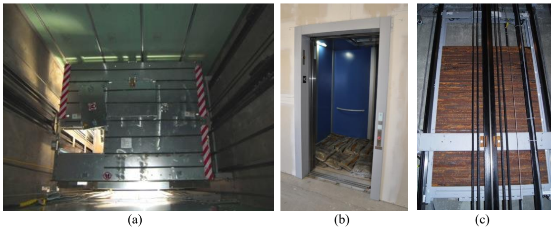
Figure 2.5: Major elevator components: (a) hoist way and top of cabin, (b) elevator doorway with sandbags inside cabin, and (c) counterweight and guiderails.
