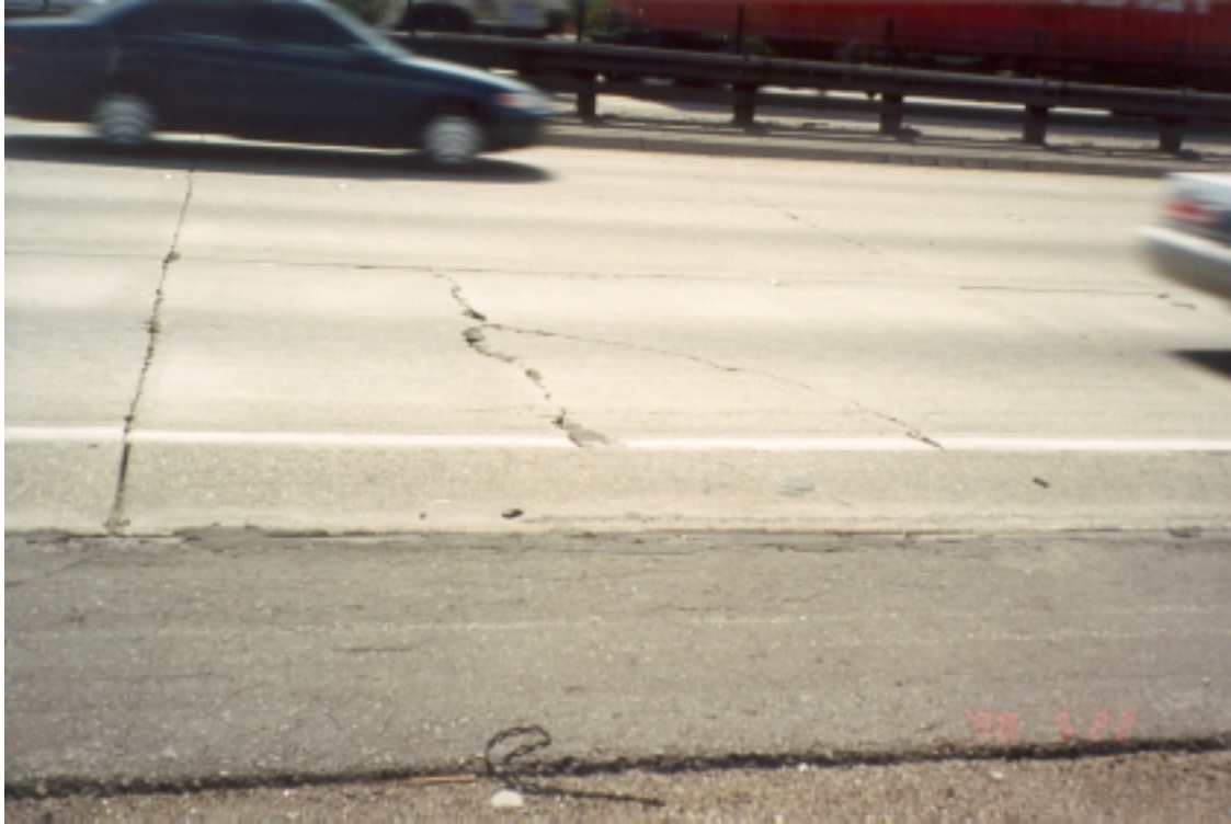
Figure 34. Pavement distress at postmile 8.3 southbound, Interstate 710: transverse fatigue cracking and badly spalled, badly faulted joint.
