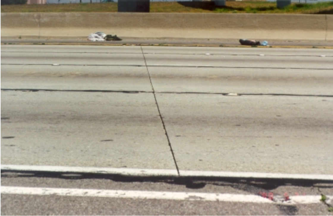
Figure 31. Pavement distress at postmile 9.6 eastbound, Interstate 10, San Bernardino county: large joint opening.
