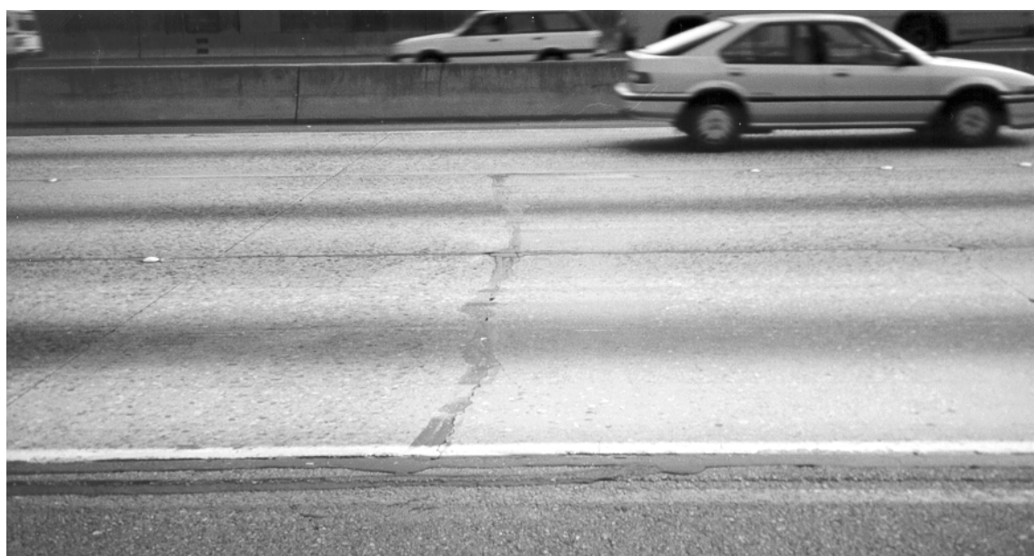
Figure 24. Pavement distresses at postmile 23.7 southbound, Interstate 5, Los Angeles County: transverse fatigue cracking and perpendicular joints.
