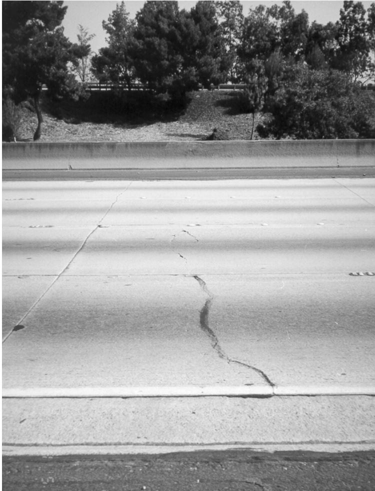
Figure 25. Pavement distresses at postmile 34.9 southbound, Interstate 5, Los Angeles County: transverse fatigue cracking and perpendicular joints.
