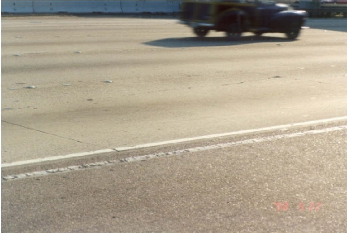
Figure 33. Pavement distress at postmile 2.7 northbound, Interstate 405, District 12: longitudinal cracking.
