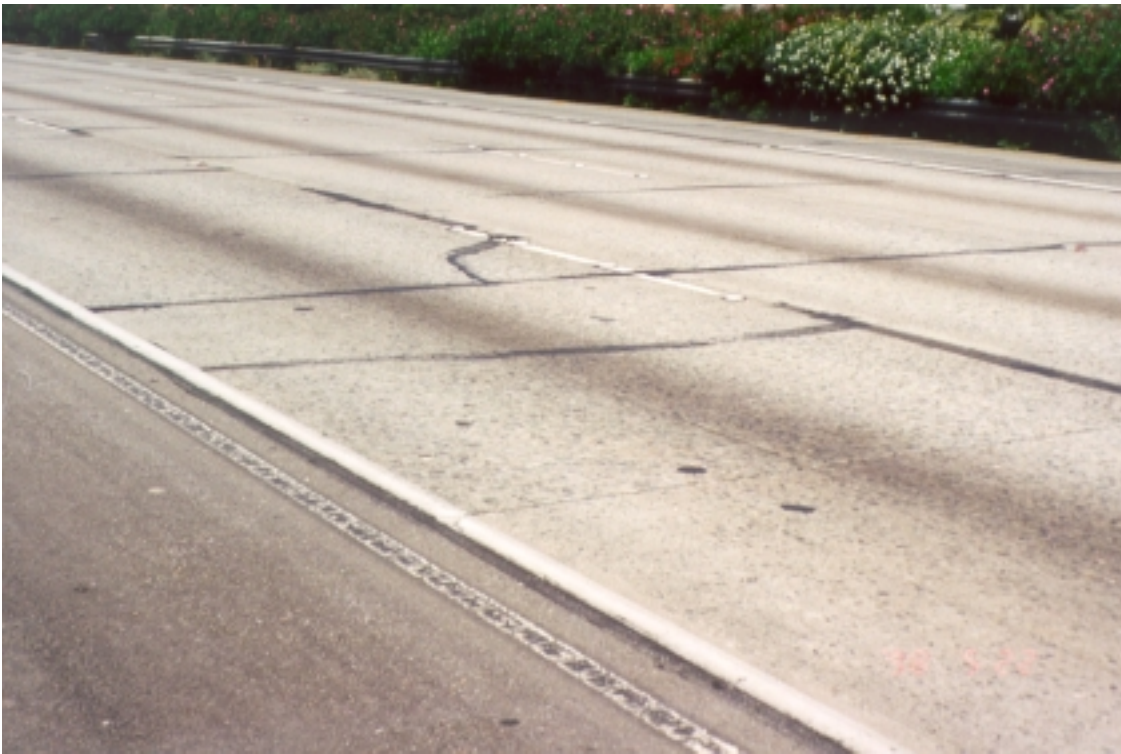
Figure 32. Pavement distress at postmile 7.7 southbound, Interstate 215, District 8: sealed corner and transverse fatigue cracking.
