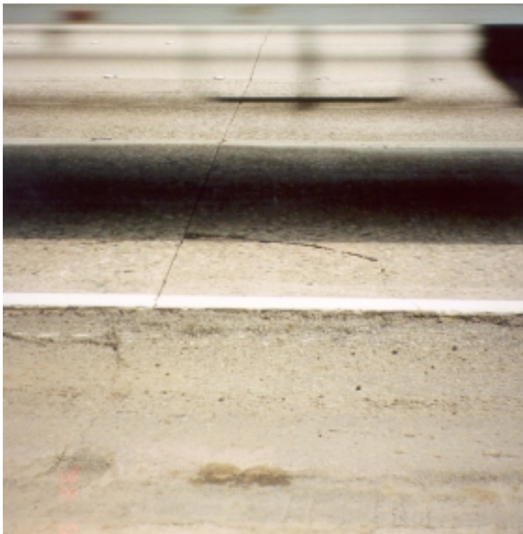
Figure 29. Pavement distresses at postmile 30.0 eastbound, Interstate 10, between Los Angeles and District 7/District 8 boundary: corner cracking.
