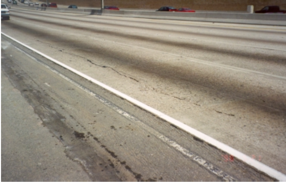
Figure 28. Pavement distresses at postmile 30.0 eastbound, Interstate 10, between Los Angeles and District 7/District 8 boundary: longitudinal cracking.
