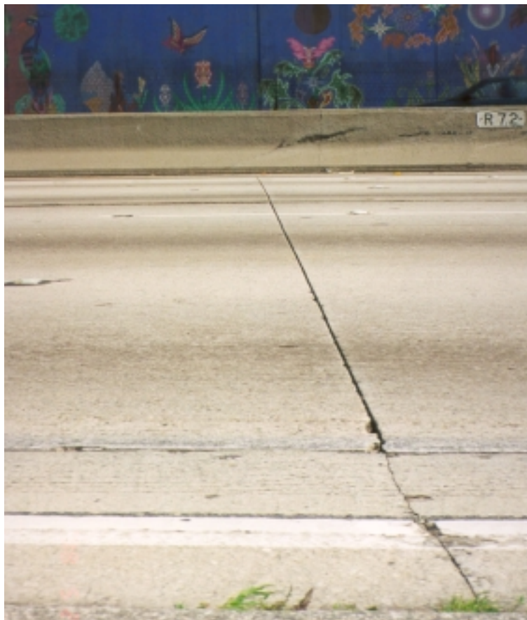
Figure 26. Pavement distress at postmile 12.9 westbound, Interstate 10, between Los Angeles and District 7/District 8 boundary: large joint openings, faulting, no cracking.
