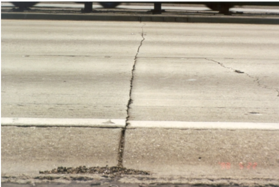
Figure 35. Pavement distress at postmile 8.3 southbound, Interstate 710: spalled joint, transverse fatigue cracking.
