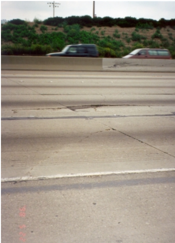
Figure 36. Pavement distress condition at postmile 17.3 westbound Interstate 60, District 7: corner cracking, transverse cracking, moderate faulting.
