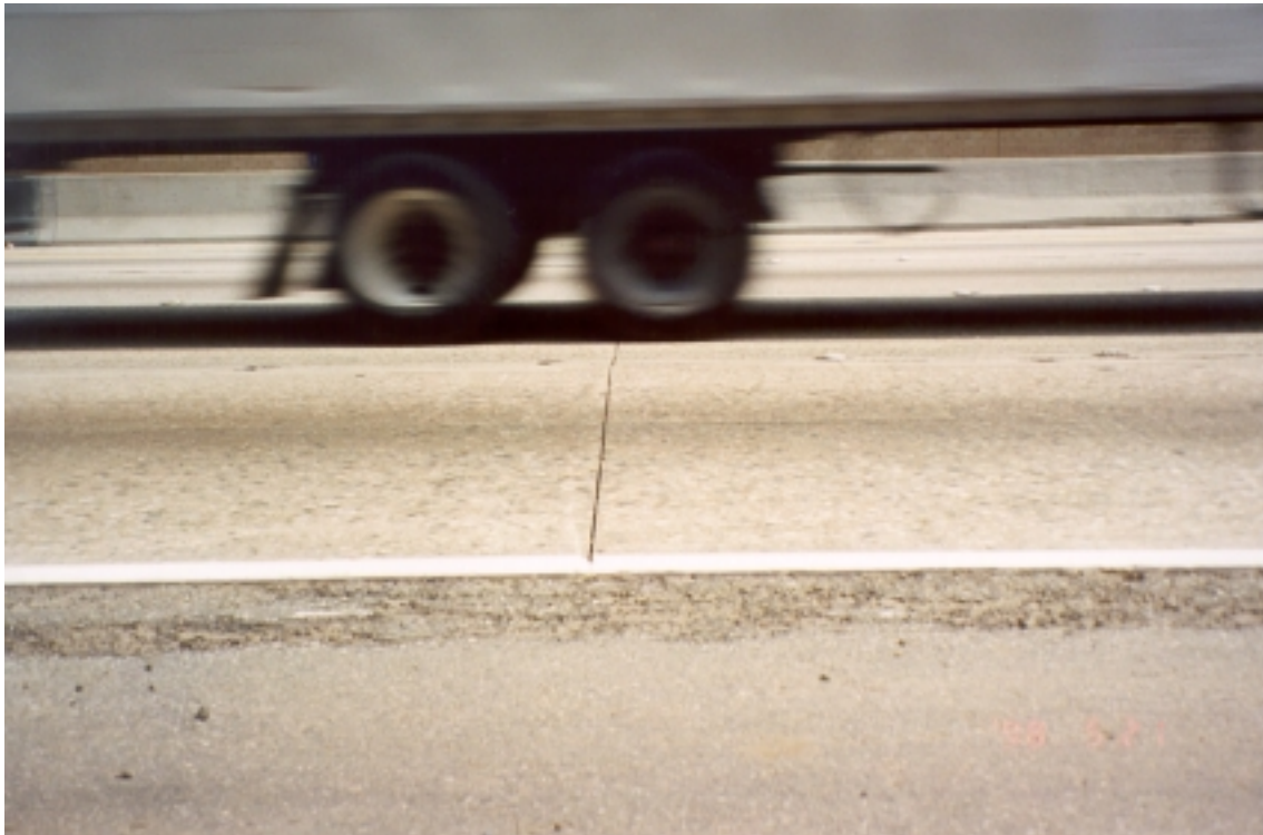
Figure 27. Pavement distress at postmile 30.0 eastbound, Interstate 10, between Los Angeles and District 7/District 8 boundary: large joint openings, no cracking.
