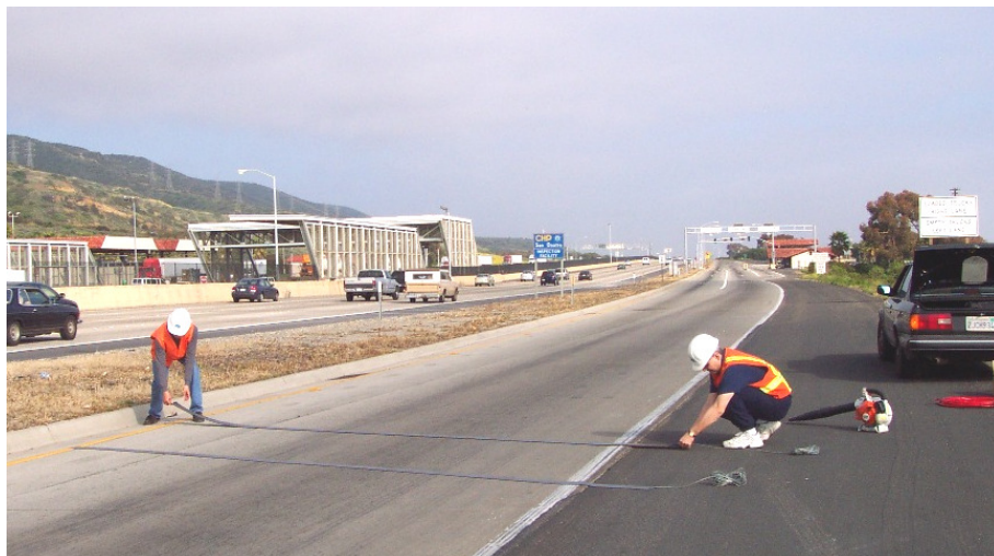
Figure 3.3. Installation of double surface-mounted Blade™ inductive sensors at the San Onofre study site
