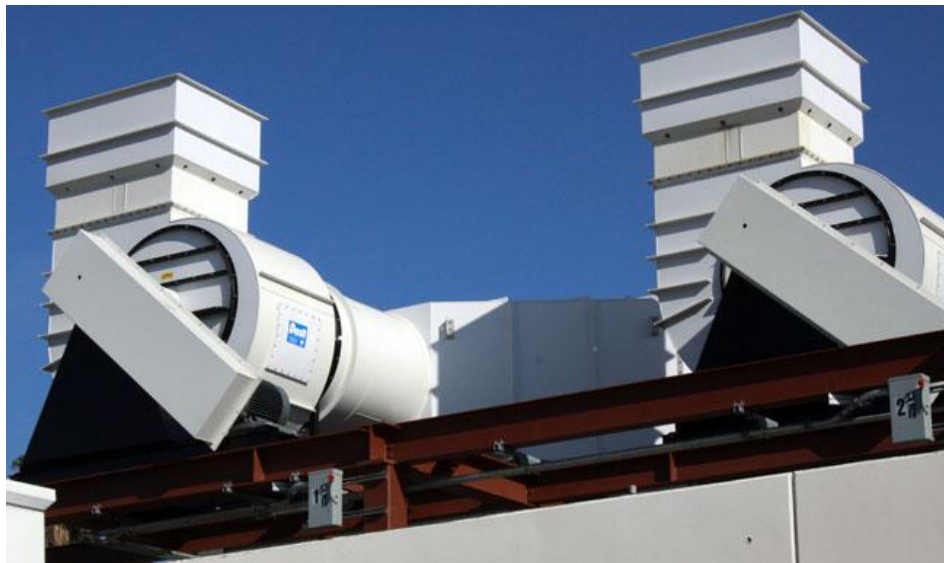
Figure 4B: Photograph of vents on top of a metal plating facility in Southeast Santa Ana
