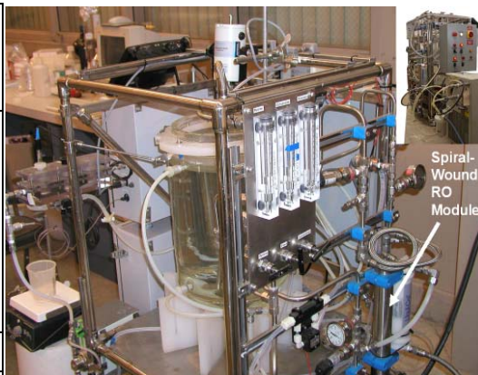
Figure 4.2. Spiral-wound RO desalination system showing RO module and degassing membrane (to the right of RO module) and crystallizer/clarifier vessel.
