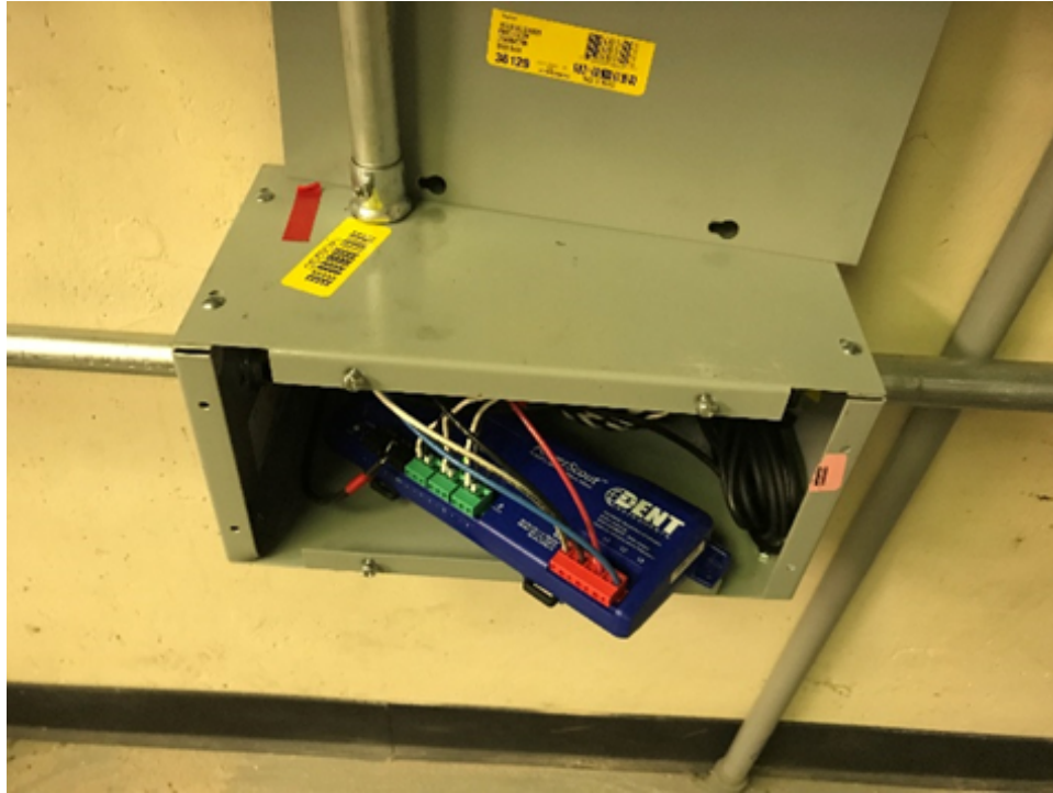
Figure 99: Franco Center DENT Power Meter Installation
