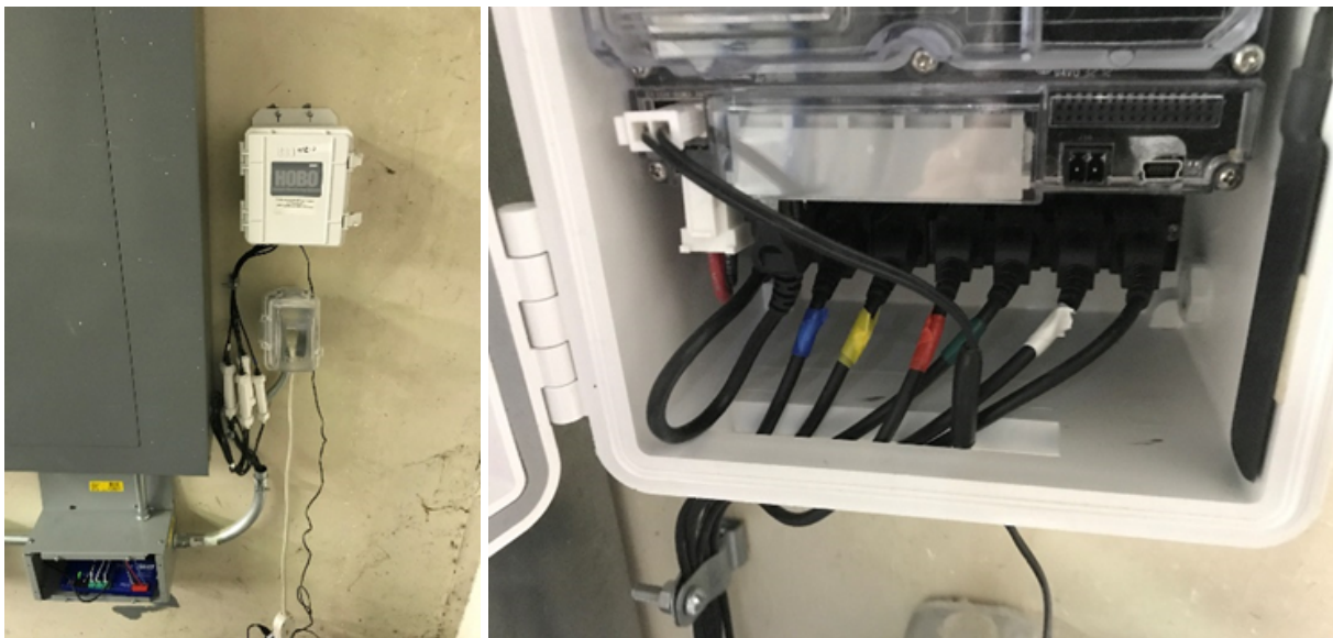
Figure 100: Franco Center HOBO U-30 Meter Installation and DENT Connection
