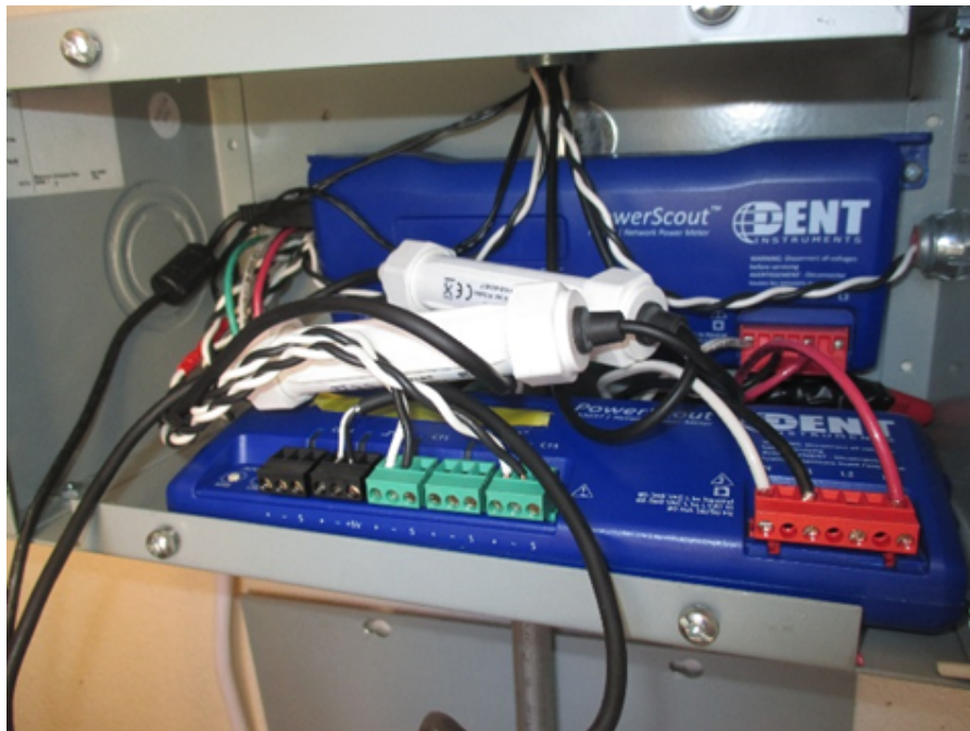
Figure 102: Rolling Hills DENT Power Meter Installation
