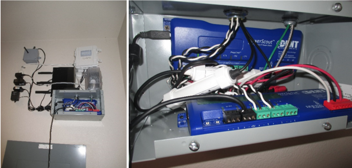
Figure 106: Parksdale 2 Community Building Monitoring Equipment Installation
