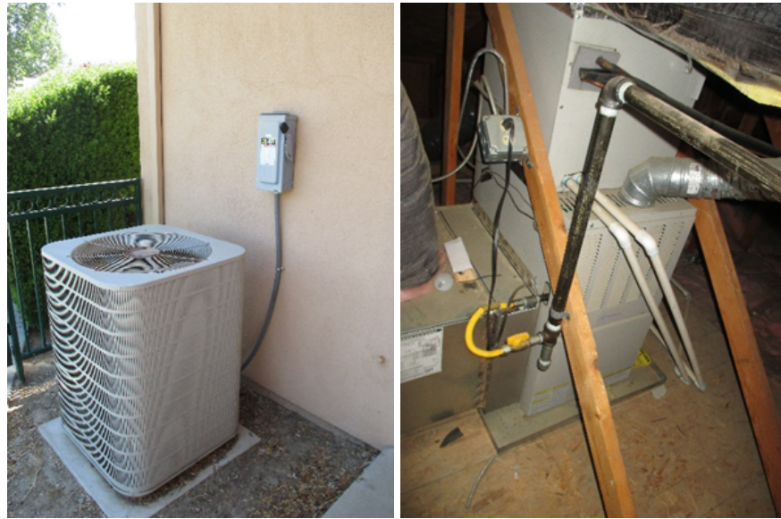
Rolling Hills exterior air conditioning condensing unit (left), and interior attic space with heating and air handling equipment (right).
