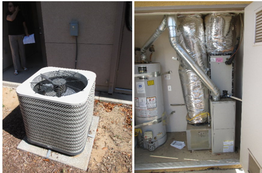
Parksdale typical dwelling unit exterior air conditioning condensing unit (left), and interior heating and air handling equipment (right).
