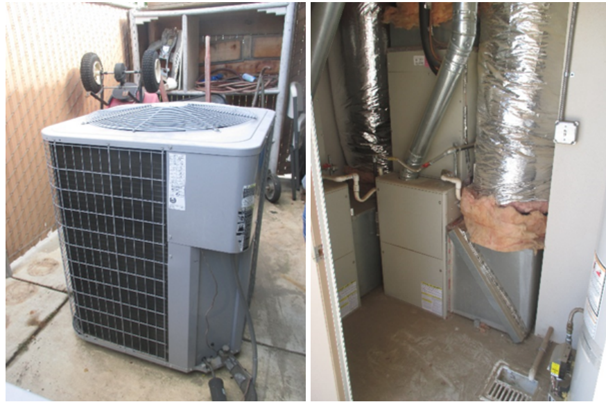
Parksdale Community Building exterior air conditioning condensing unit (left), and interior heating and air handling equipment (right).
