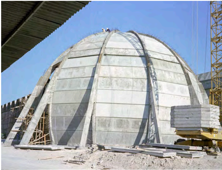
Figure 15: Photograph of the Kuwait National Museum’s Planetarium under construction. Source: Aga Khan Award for Architecture.
