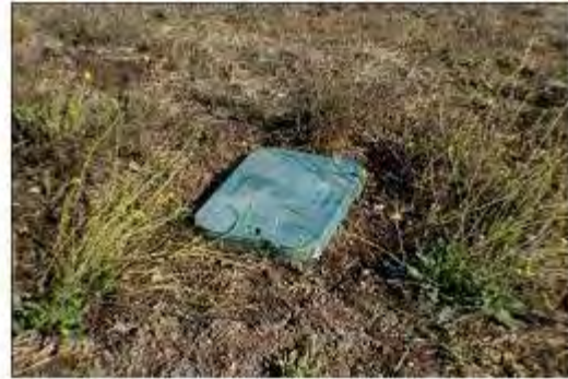
Transect 5 back shot position on electrical box
