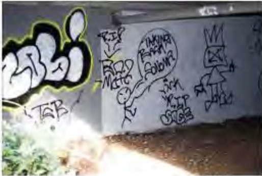
Graffiti under bridge
