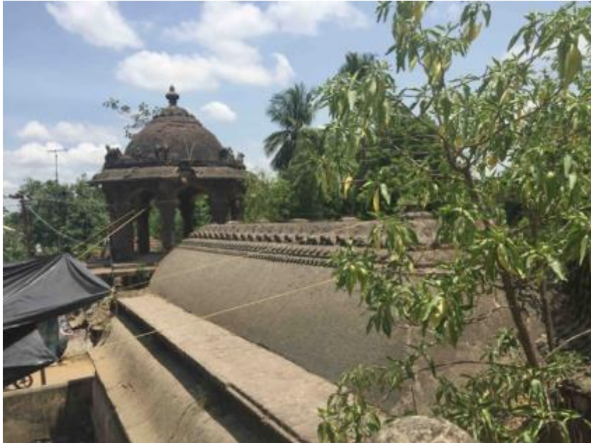
Fig. 17-18. Upper floor half roof garden of Needamangalam Yamunambal chatram. Photographs from author's travel.
