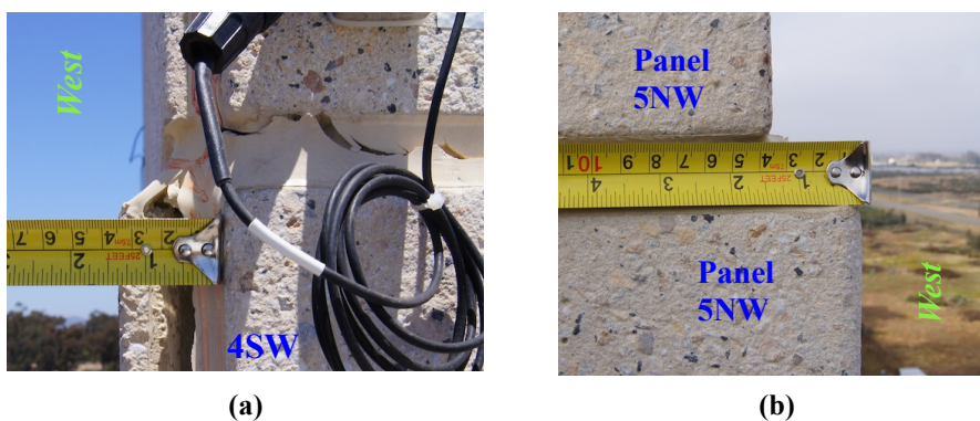
Figure 3.18. Misalignments of the panels at the fourth level in the (a) SW and (b) NW corners
