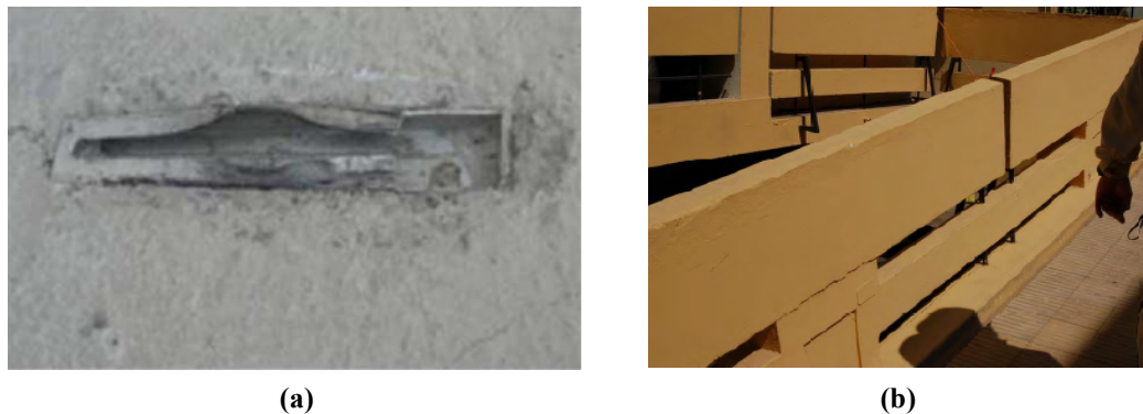
Figure 1.16. Damage to APC panels during the 2010 Maule earthquake: (a) damage to cladding connection (Gosh and Cleland 2010) and (b) damage to railing panels (FEMA E-74 2011)
