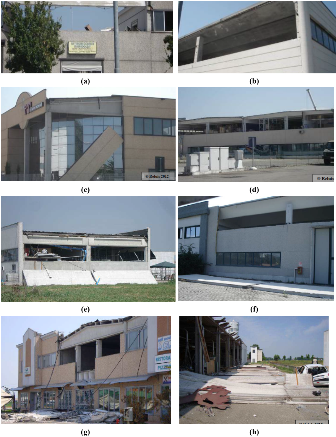
Figure 1.20. Building that experienced collapse of roof and APC cladding during the Emilia earthquake (Ercolino et al. 2012a, Ercolino et al. 2012b, Di Croce et al. 2012)
