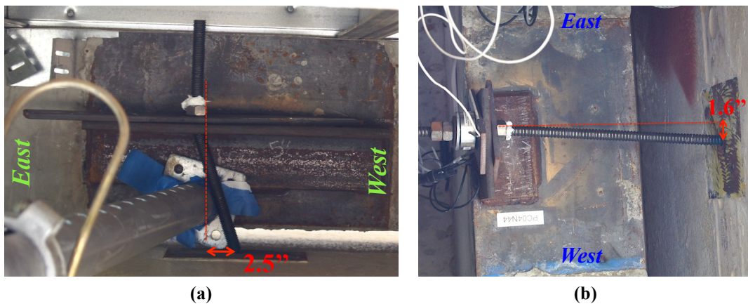
Figure 3.14. Damage to tiebacks after FB6: (a) connection CE in panel 4SW and (b) connection EE in panel 4NE
