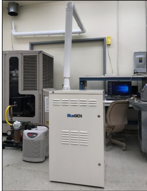
Figure 5-1: 1.5 kW BlueGEN installed in the NFCRC laboratory
