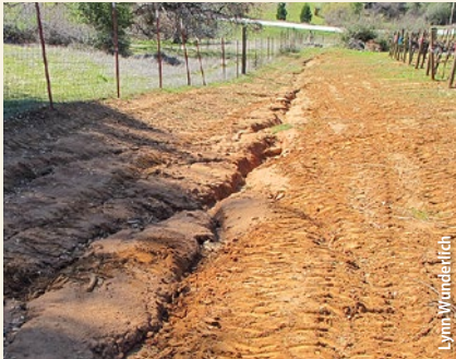
Sheet and rill erosion on an unimproved dirt road. Rills are the channel networks. Areas of sheet erosion are the smooth textured surface soil surrounding the rills.
