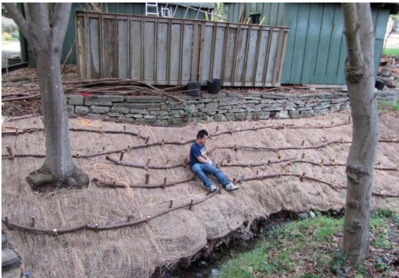
Figure 3. A student stakes down a geotextile fabric on the northern bank of the upper reach of Cerrito Creek within Blake Garden. Upper reach of Cerrito Creek Phase 1 restoration, February 2012 (Blake Garden).
