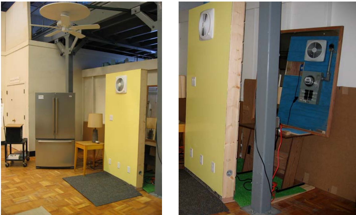
Figure 109: Left: “The Wall” demonstration test bed. Right: Watt-hour meter and breaker panel shown in mirror.
