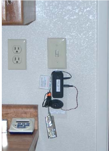
Figure 39: Example of generic mote installation.
