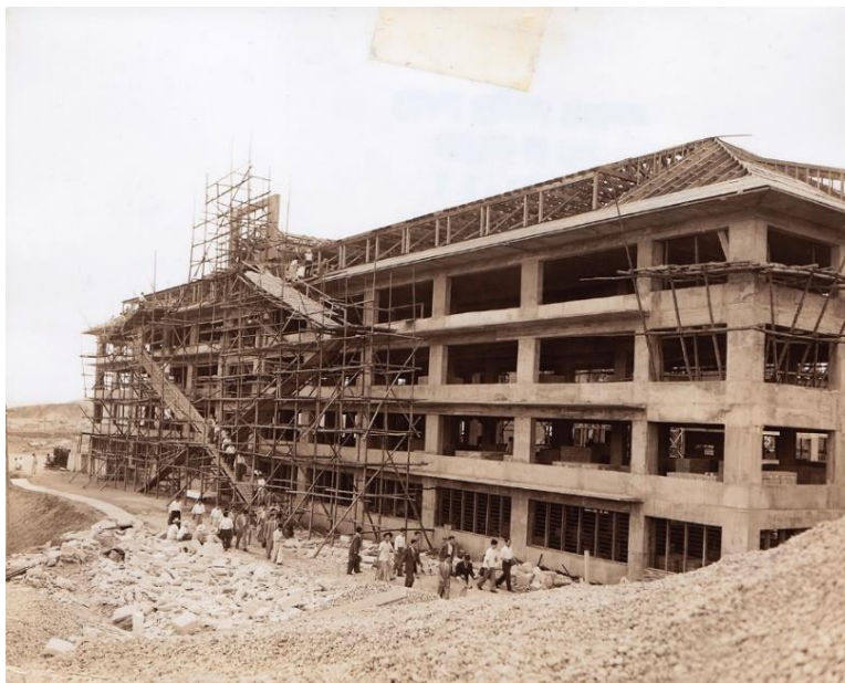
Figure 3.3 The Memorial Chest Hospital under construction, Seoul, June 12, 1956 (source: Records of the Office of the Chief Signal Officer, Research Group 111-SC; National Archives at College Park)
