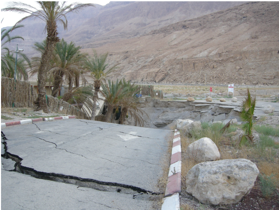
Figure 1. The new sinkhole. Photo by author, 2015.
