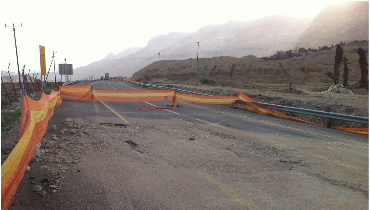
Figure 28. Repaved section of Route 90 that remains closed because of sinkholes. Photo by author, 2015.
