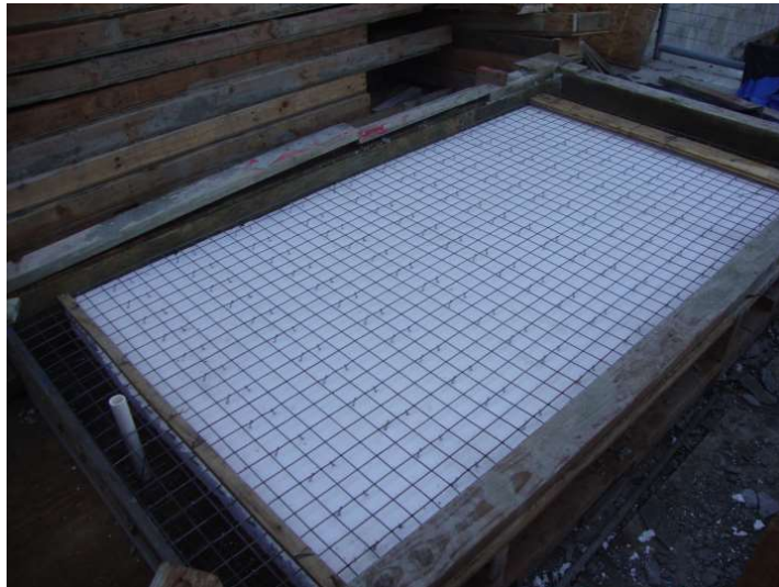
Figure (2.7): EVG 3D Panel Slab Speciment prior to Mortar application at UCI [11]
