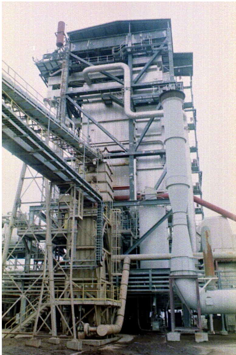
Figure 5A. The central boiler stack of the commercial biomass plant used by Jenkins et al. (1999) for controlled fuel intake experiments. Fly ash produced as part of this experiment was used in the present study.
