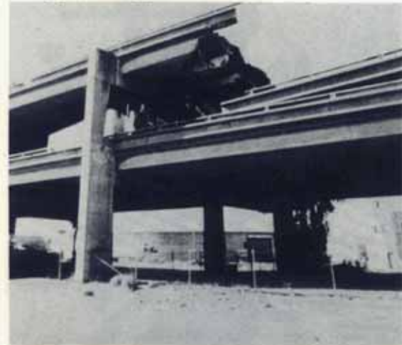
Damaged section of Oakland Cypress structure.
