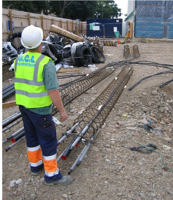
Figure 4: Loops installed within 10 m cage for 20 m deep piles at Westminster Academy
