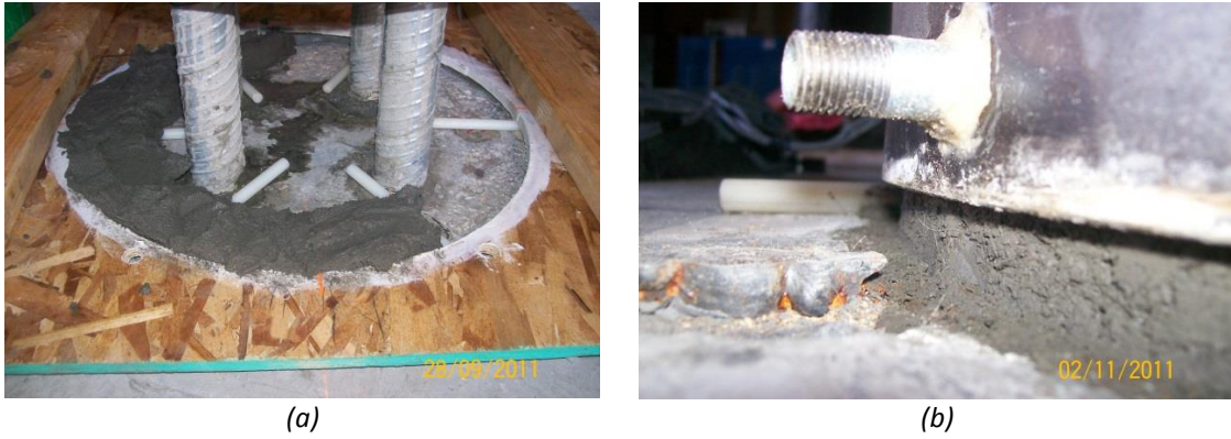
Figure 3.5 – Mortar bed: (a) wood template and nylon-rod shims, during mortar placement; (b) mortar scraped from underneath the outer shell.
