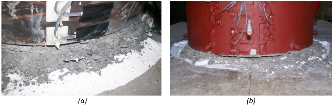
Figure 3.20 – Crushed mortar bed at the end of testing: (a) Unit 1A; (b) Unit 1B.
